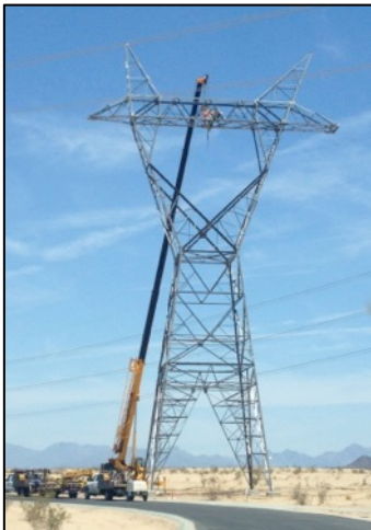
Devers-Palo Verde 2 Transmission Line in Riverside Co, California
