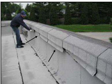
Entire cap flashing has failed in the area above the interior leak. Improper cap flashing. This is happening around the entire building perimeter. A metal cap should have been used.
