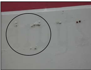
Grid location B6 - Improper patch from old sign.
