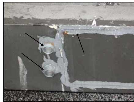
Grid location B6 - Old sign race way on roof not been removed. Conduit openings are exposed and access panels are not sealed. This is allowing water entry.
