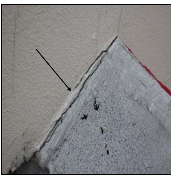
Cracks allowing water in to wall.
