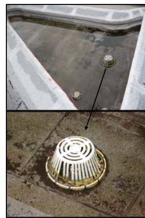
Standing water with drain photo showing drain sitting higher than the roof.
