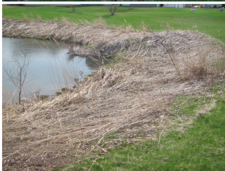
Missing plantings along Stormwater Management Area South
