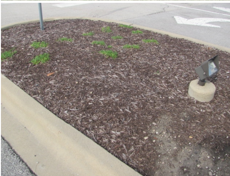
Missing plantings at Renwick Road and Crossing Drive entrance
