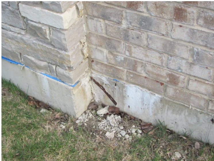
Exposed anchor at Renwick Road and Cove Circle entrance monument
