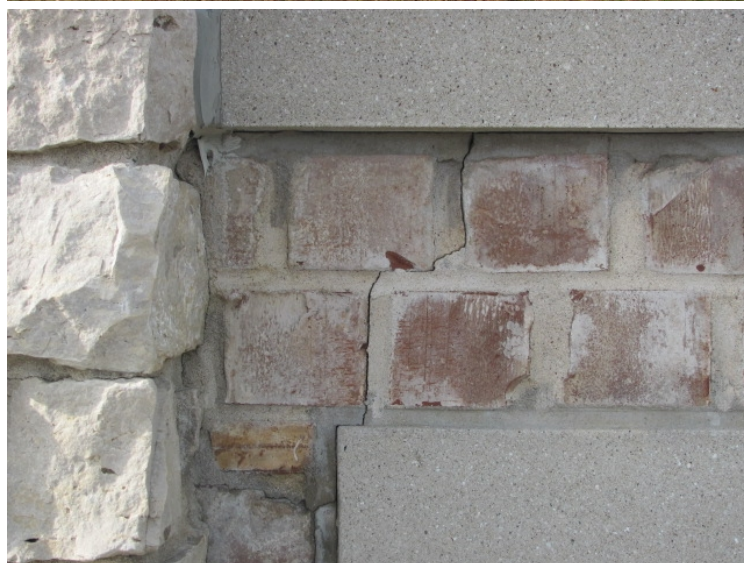
Step crack at Renwick Road and Creekview Drive entrance monument
