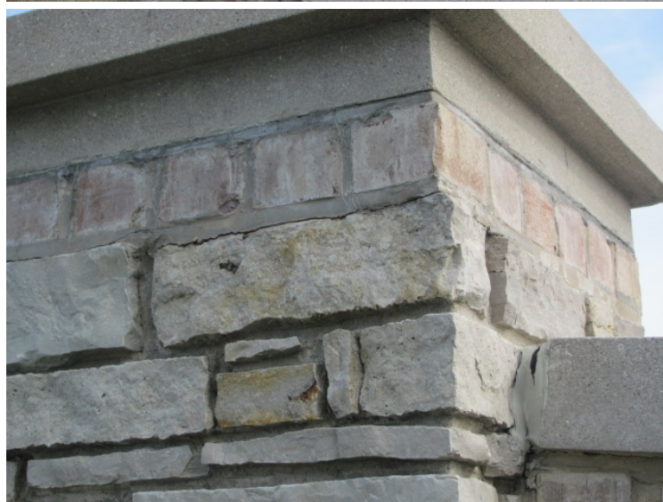
Mortar crack at Renwick Road and Cove Circle entrance monument
