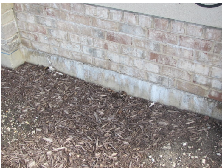
Efflorescence at Renwick Road and Crossing Drive entrance monument
