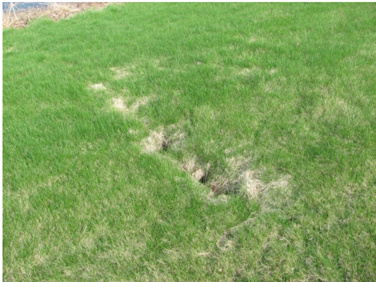
Erosion along west side of Stormwater Management Area South
