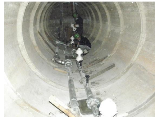
Inside of aeration tank
