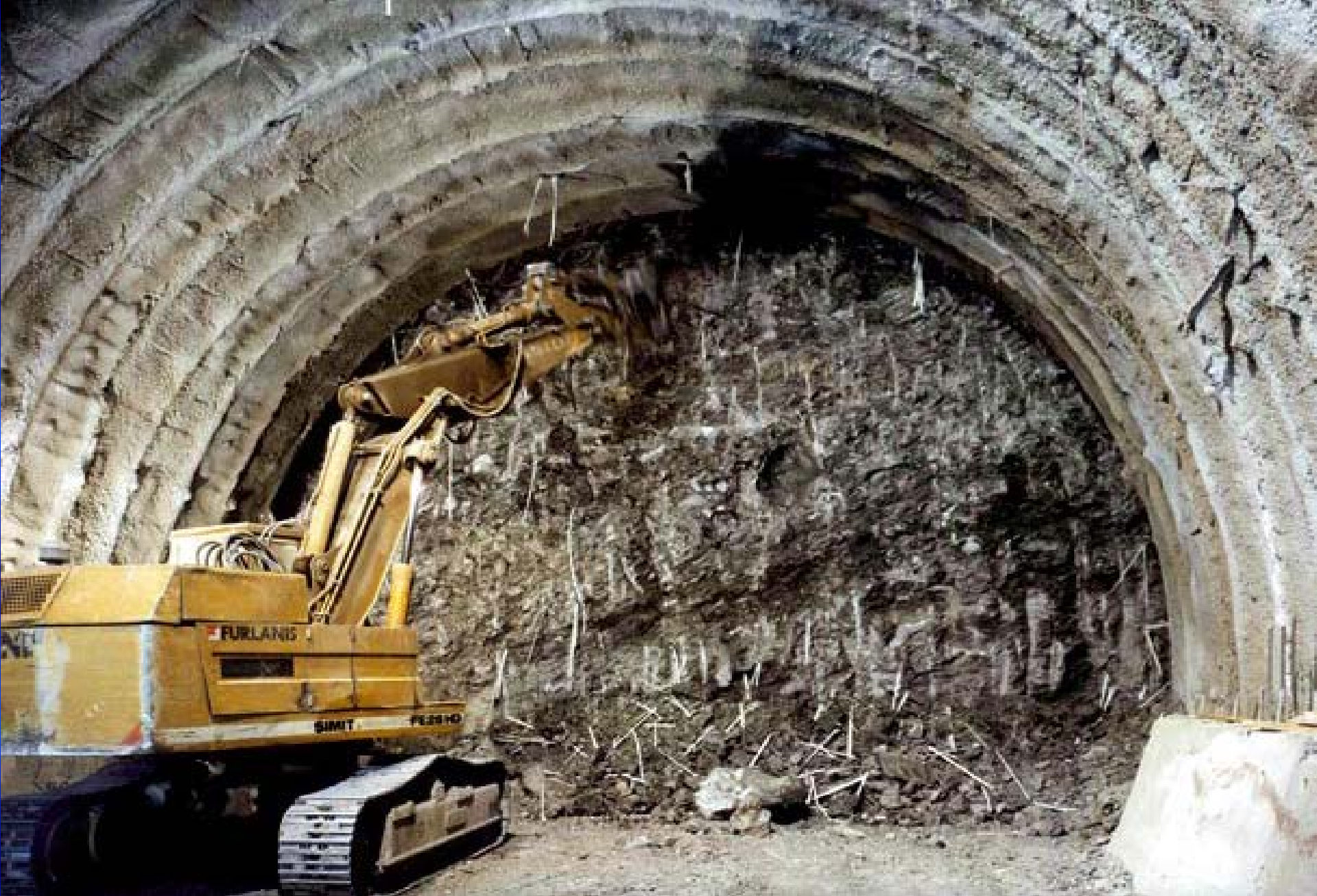
San Vitale tunnel - Caserta-Foggia railway line. Ground: scaly clay. Overburden: ~ 130 m. Face reinforced with fibre glass structural elements . [Lunardi Project]
