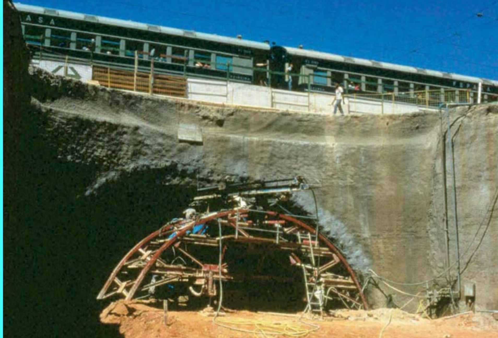
View of the portal constructed using a shell of ground improved by means of jet-grouting and face reinforced with jet grouting elements. In Campinas (Brazil) [Lunardi Proyect]
