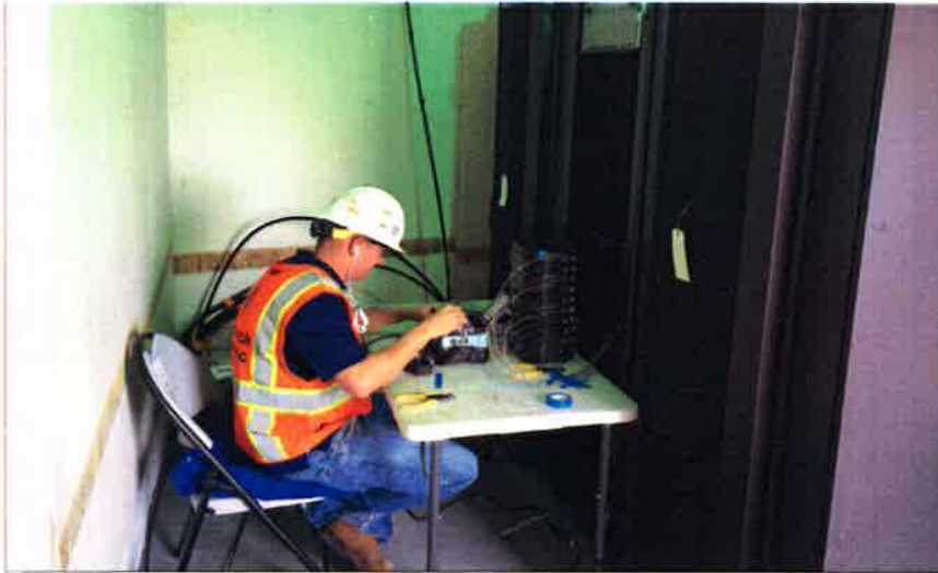
RSS SLDCA IT Room Fiber Splicing
