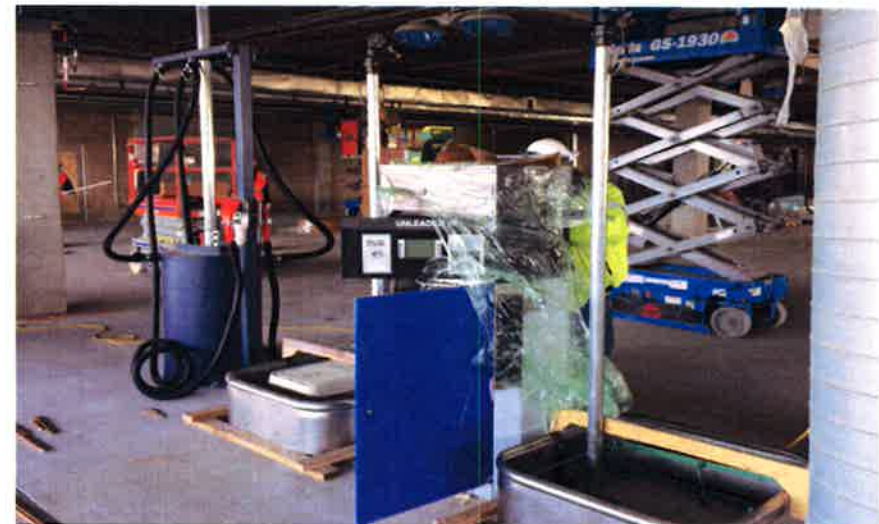
Pre-Functional Check for Fueling System
