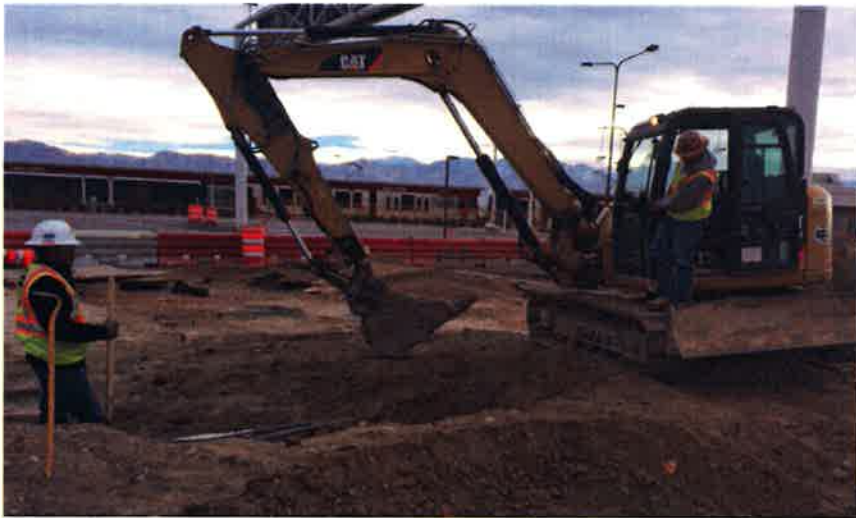
East Lift Station Piping across the Entrance Road.
