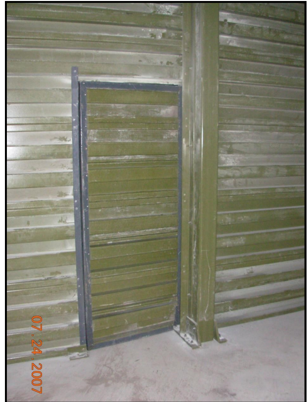
Rear View of access door at St. Cloud, FL
