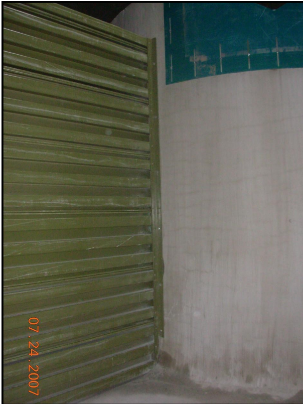
Clearwell Baffle Wall and round concrete tank at St. Cloud, FL
