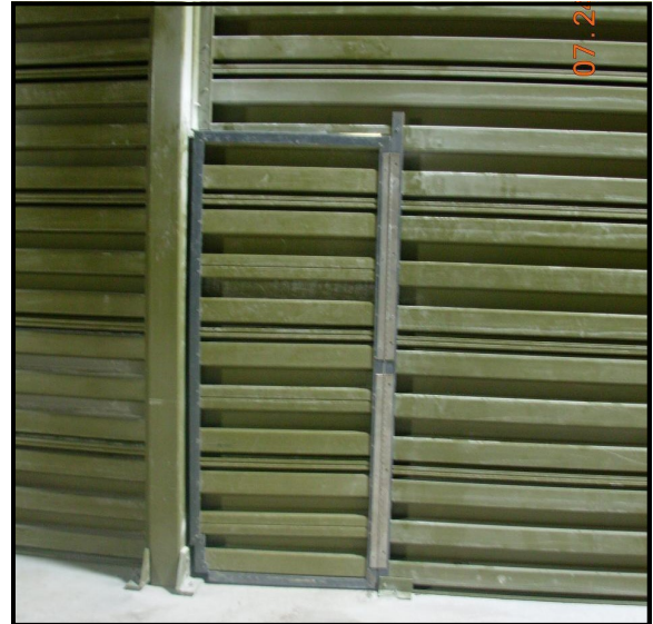
Access door in Baffle Wall showing hinge connection on opening side at St. Cloud, FL
