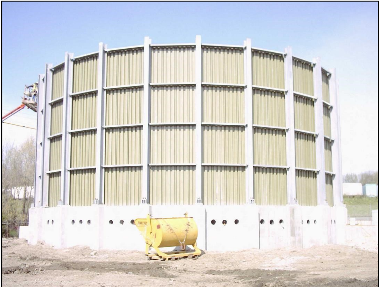
Trickling Filter at Leavenworth, KS using baffle panel in vertical position with batten strips over seams.
