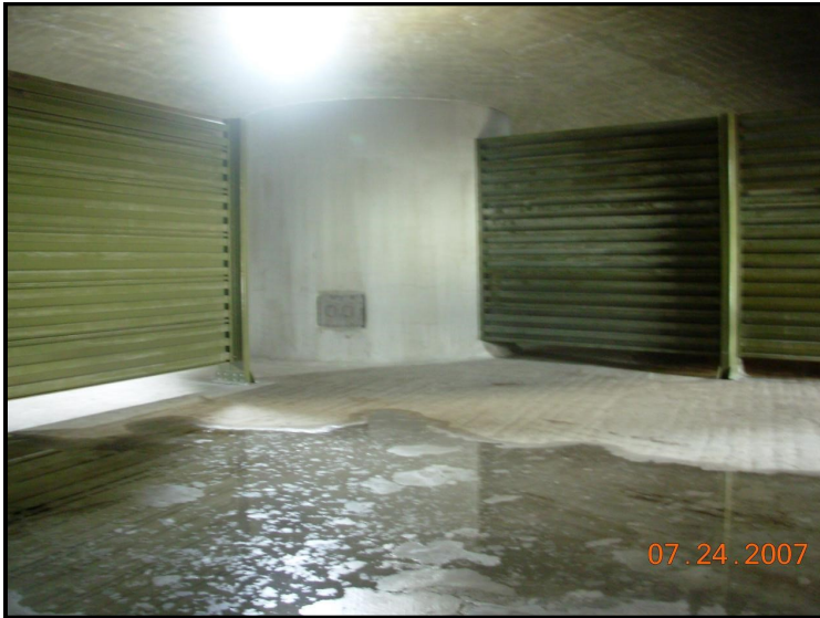
Fiberglass baffle walls in Clear Well at St. Cloud, FL
