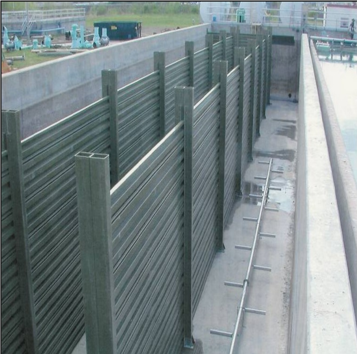
Chlorine Contact Basin at Keegan's Bayou WWTP, Houston, TX
