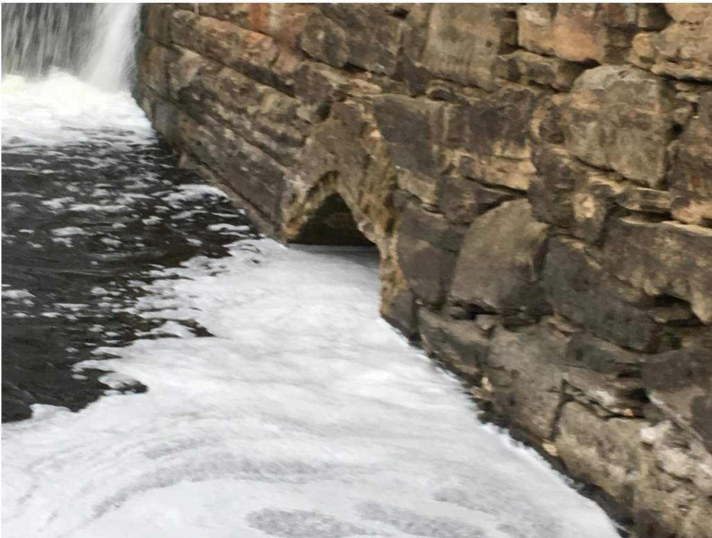
Photo 23 – November 28, 2016 View of Scott's Mill Grist Foundation (Left Abutment) Showing Grist Mill Discharge Location
