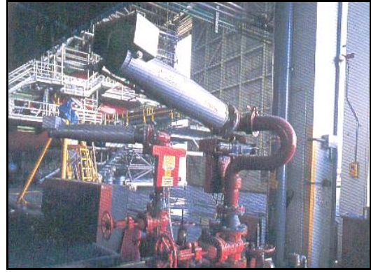
Fire equipment in the new hangar
