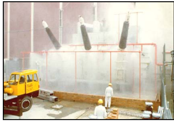
Wallerawang Power Station, Transformer protection
