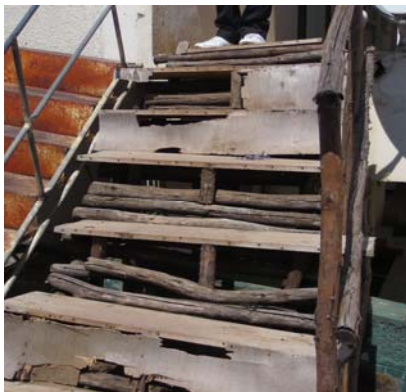
Steps in need of repair!
