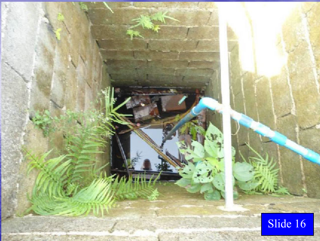
Photo 3: Neglected Well unsecured and accumulating Trash
