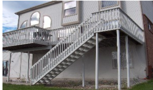
Old, unsafe deck
