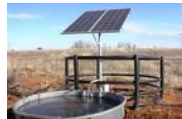
Solar PV Water Pumps
