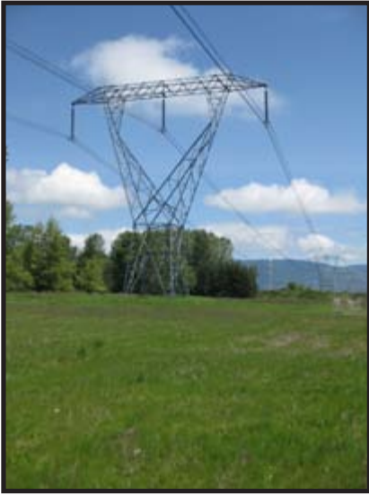
BPA electrical transmission lines
