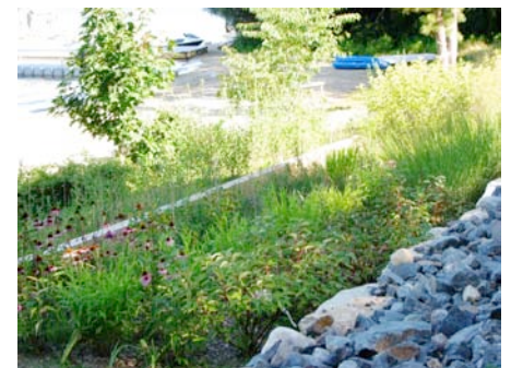
Rain garden installed by the Town at as part of the Shore Rd. Project
