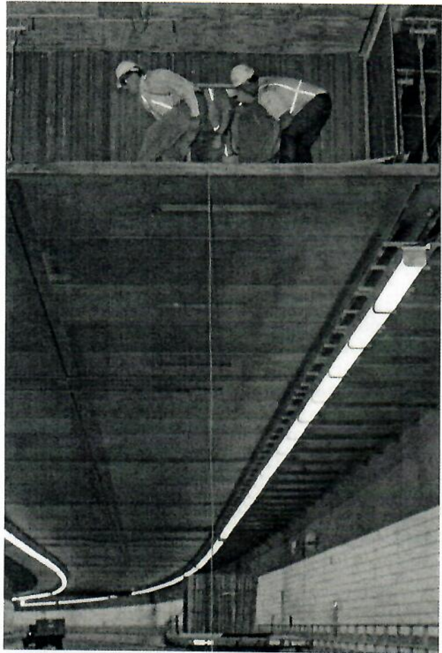
Then-Governor Mitt Romney inspecting a roof that collapsed in "the Big Dig"—the tunnel under downtown Boston.
