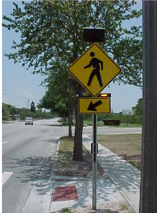
Figure 1. Photo. RRFB with two forward-facing LED flashers and a side-mounted LED flasher.
