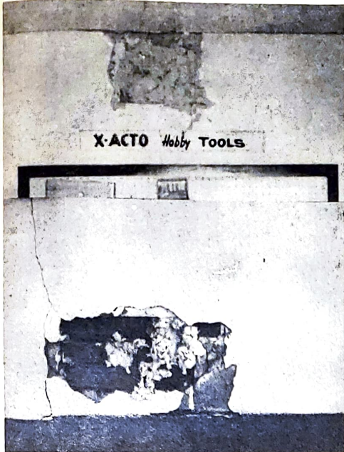
The above picture shows the damage made by the three men attempting to enter Pascals Hardware early Sunday morning. It appears that the would-be thieves would have had considerable difficulty making good their entrance as their hole was at the top of a deep stair well.
