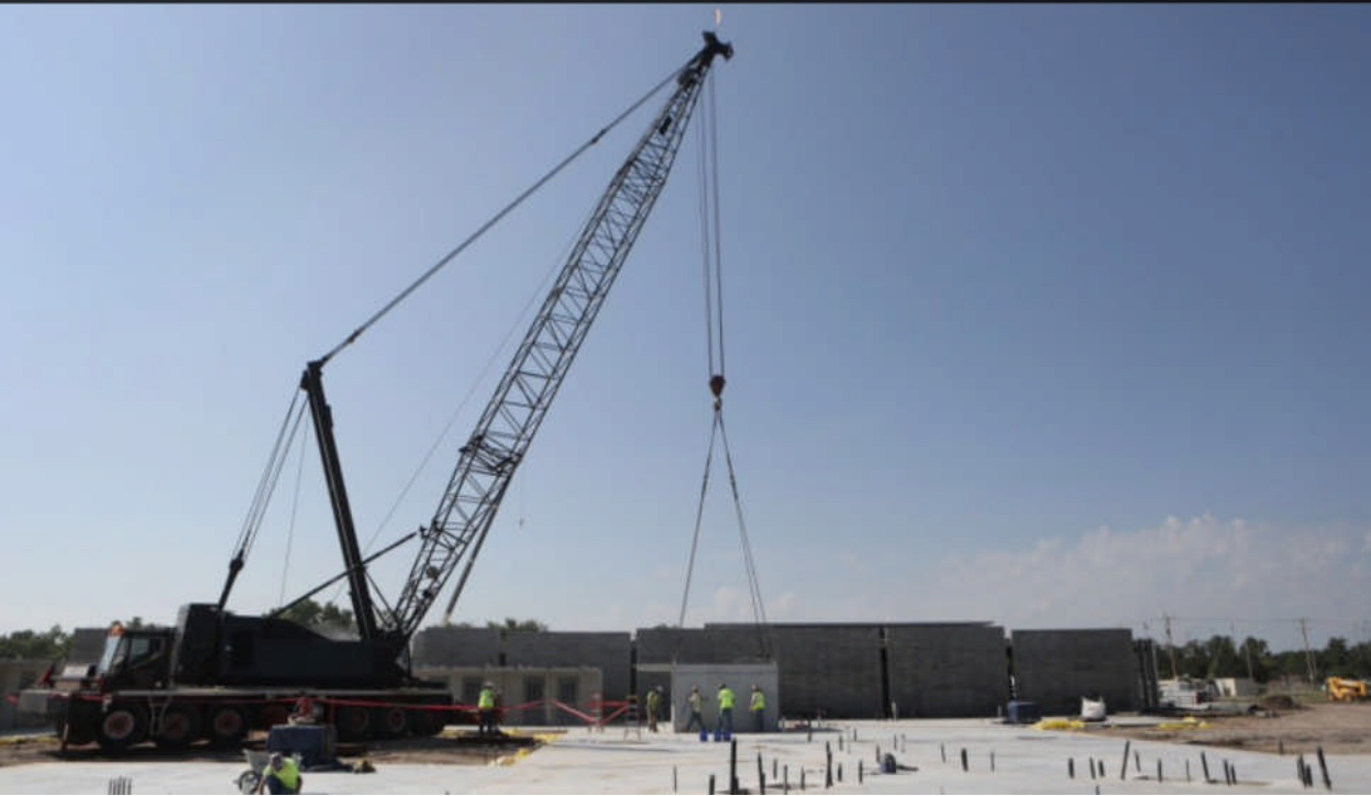
New Jail: Construction of the new Reno County Jail, expected to be finished in June and will host inmates as of August 2015. - Megan May/The Hutchinson News
