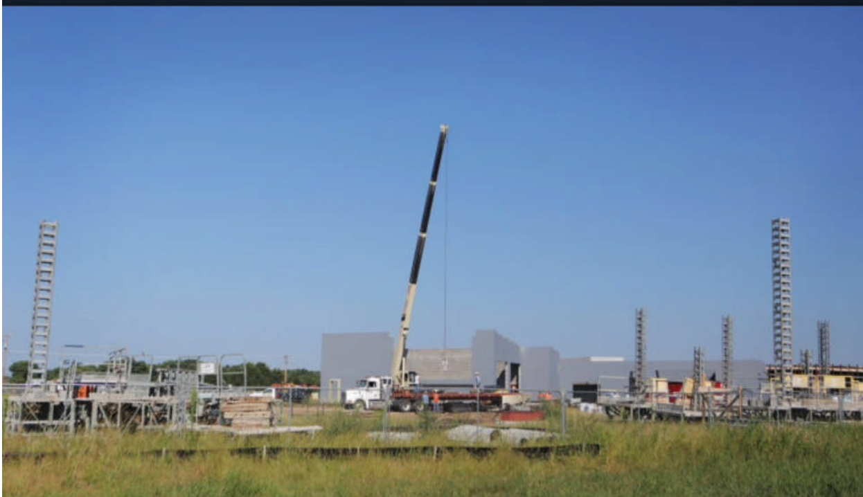
New Jail: Construction site of the Reno County Jail in Hutchinson on Wednesday, Aug. 20, 2014. - Megan May/The Hutchinson News
