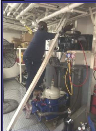
Hughes Technician Dave Smith replaces a leaking combination sight glass and drier on the Freezer Condensing Unit
