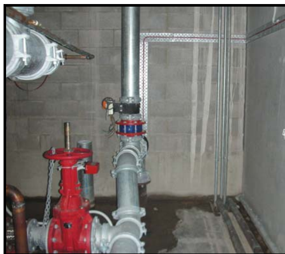
Figure 6 – Pump Room Leakage
