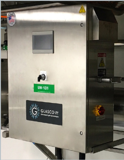
Remote Ballast Control Center (BCC) houses ballasts, controls, monitors and PLC.
