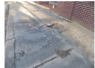
Interrupted sidewalk @ 1 st Street & N. Boyce Lawton Drive
