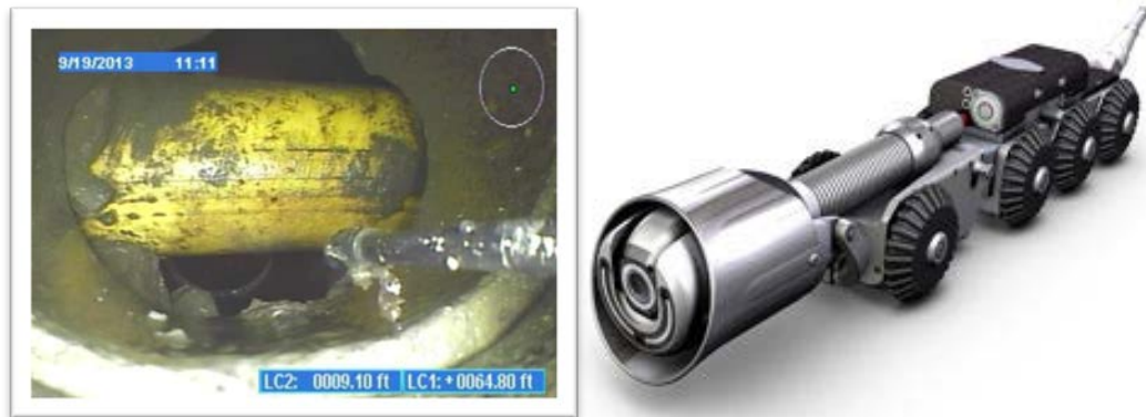
Figure 2. CCTV sewer inspection with a rugged remote controlled lateral launch camera collects evidence that identifies gas cross bores or verifies their absence.
