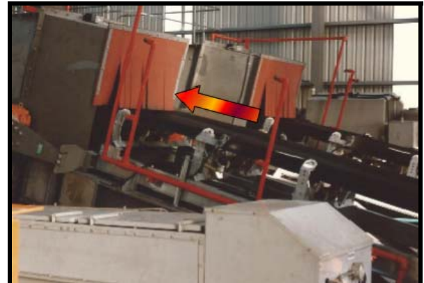
Figure 5 - Conveyor Head protection
