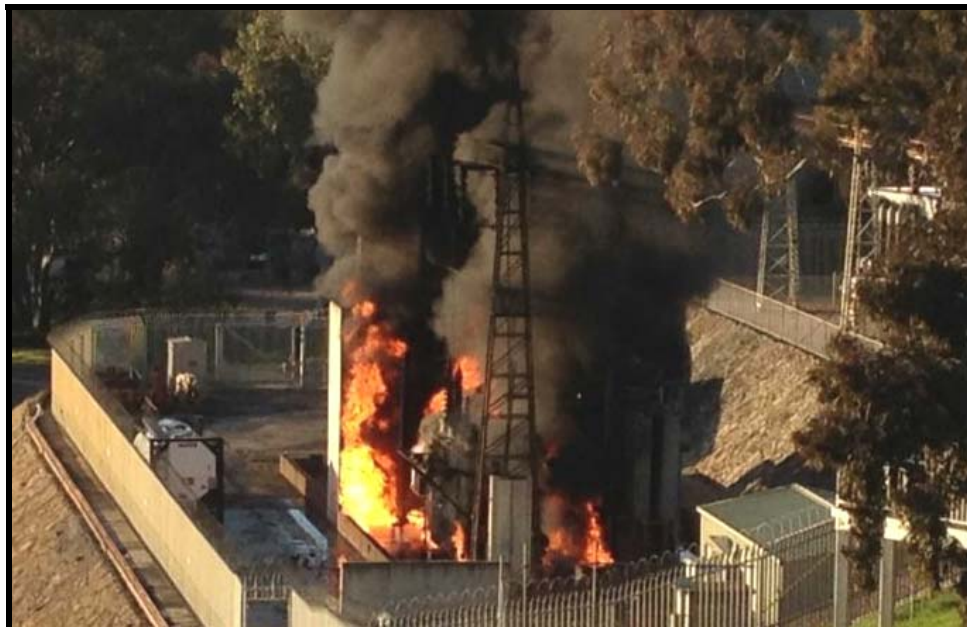
Figure 2 – Hume Weir Transformer Fire
