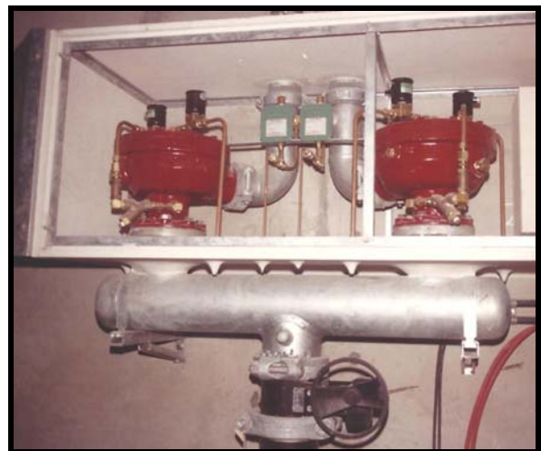
Figure 28 - Sydney Harbour Tunnel Deluge Valves
