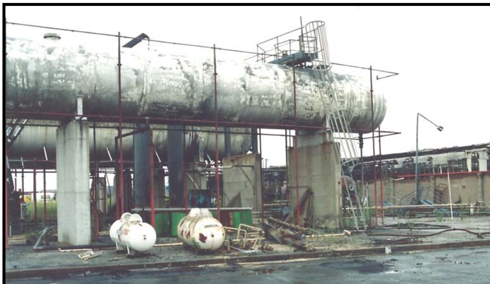
Figure 6 – Results of a LPG Tank Fire
