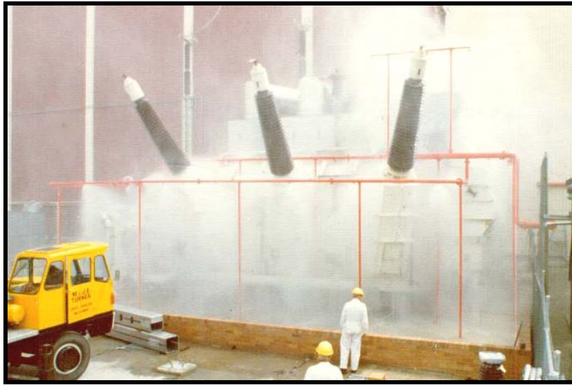
Figure 3 – Wallerawang Generator Transformer Waterspray System
