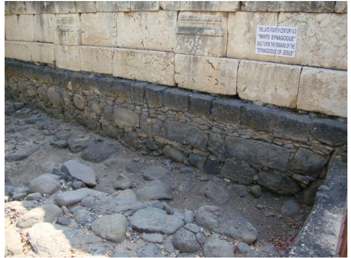
The Basalt / Volcanic Rock Foundation from the First Century Synagogue, the Black Rock is shown above
