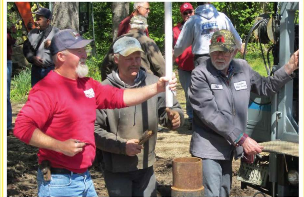
Ross Deschaine of Sunco, left, with Scott and Skip Hodgdon, right, of Hodgdon Well Drilling of Poland work on the installation at the Robert's Farm in Norway for the MGWA Spring Demo. The Hodgdon's donated the well. See Story Page 2.
