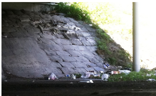
The contractor had not been maintaining the area.
