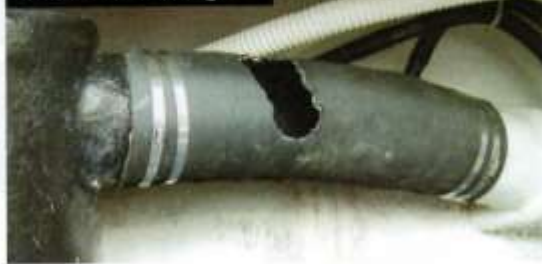
Exhaust Hose Damage
