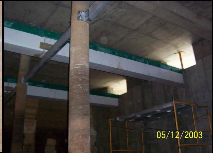
Rocklin, CA troughs fixed one end supported by steel beam on other end.
