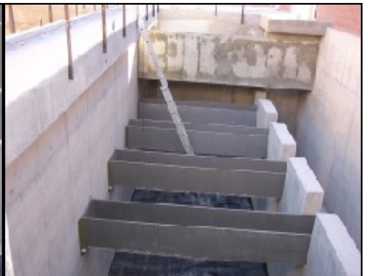
Chalk Bluff, NV troughs anchor bolted to effluent end.
