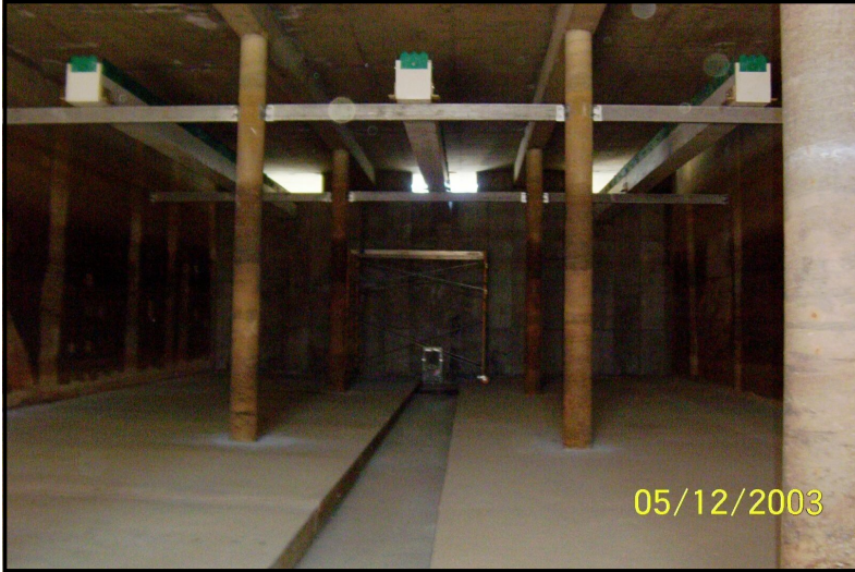
Rocklin, CA troughs supported on steel beams. 12" wide x 18" deep trough spanning 24'0" Ends not fixed
