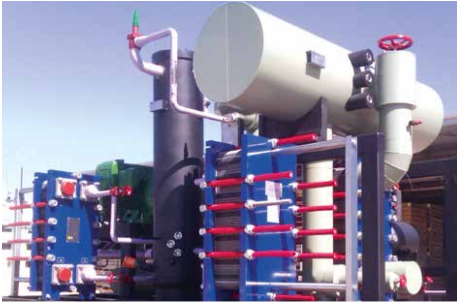
The Ammonia plant at Parilla, which was a finalist in 2014 AIRAH Awards' Best HVAC&R Retrofit or Upgrade category.
