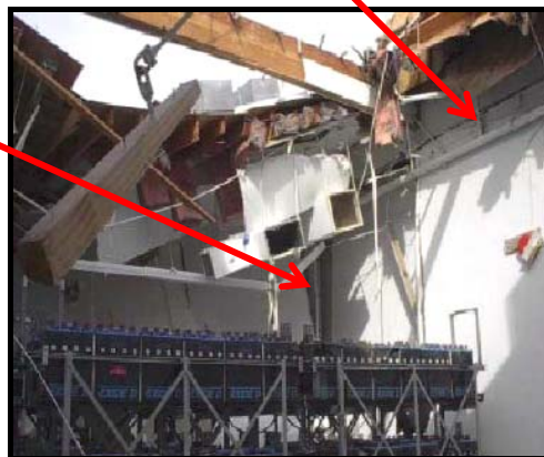
Figure 17 – Battery Explosion Results
