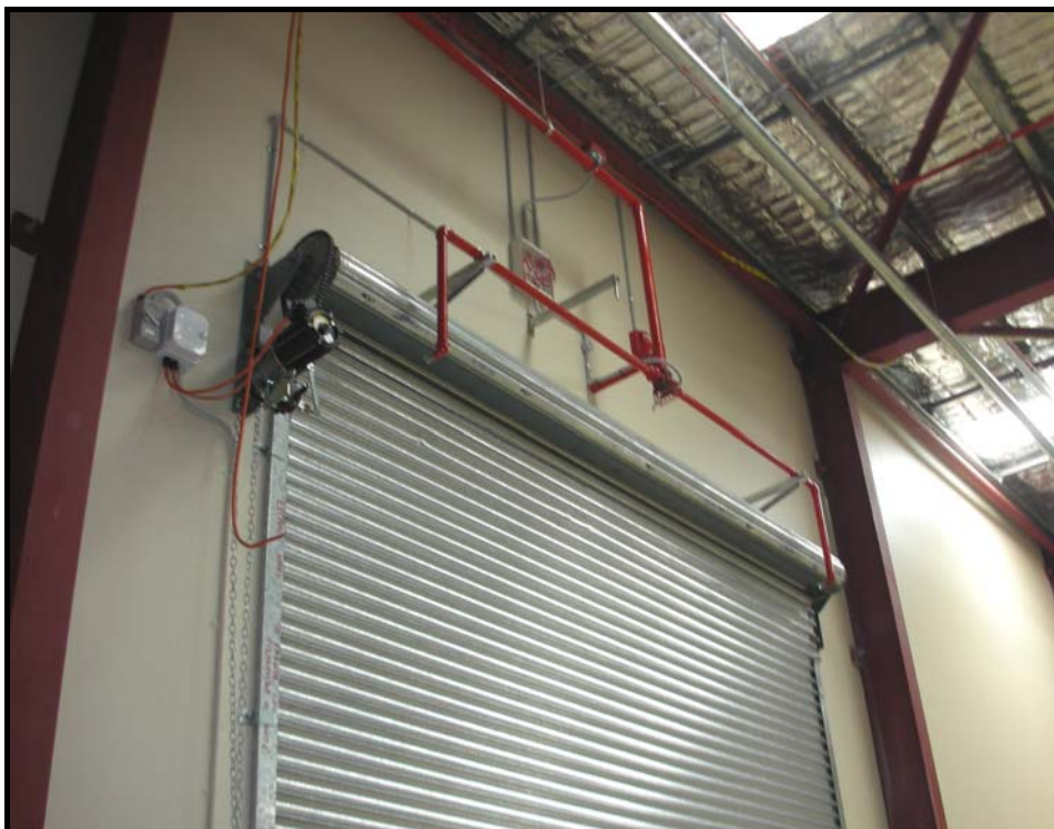
Figure 21 – Drenchers on Roller Shutter
