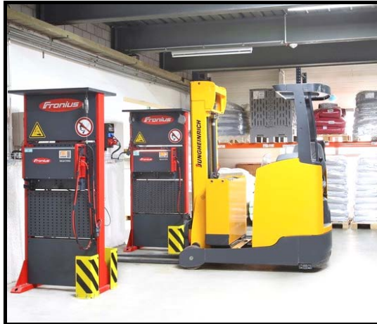
Figure 22 – Distributed Charging Station
