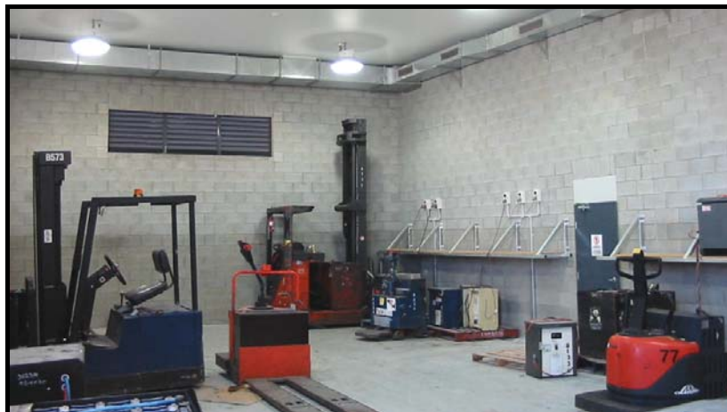
Figure 6 – Typical Battery Charging Room –
