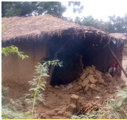
One of our staff's homes. With driving rain day after day... mud bricks put together with mud mortar disintegrate, the lower areas soften and the weight of the wall results in collapse.
