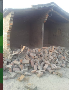
Another of our staff's houses, bedroom and storage room open to all... now to repair/rebuild.
