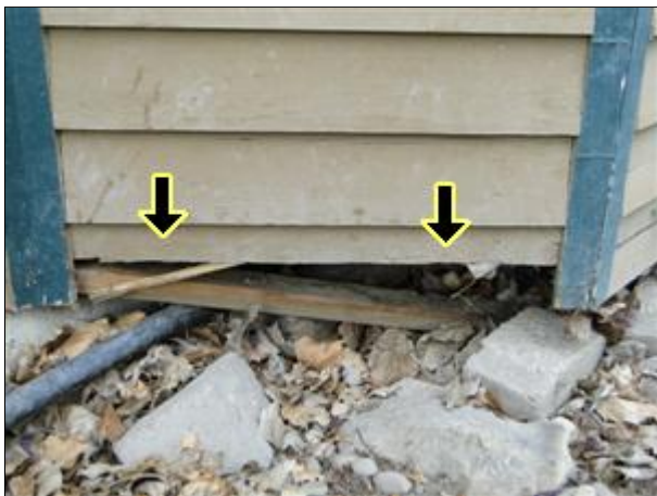
2.1 Picture 3 Damaged cladding board.
