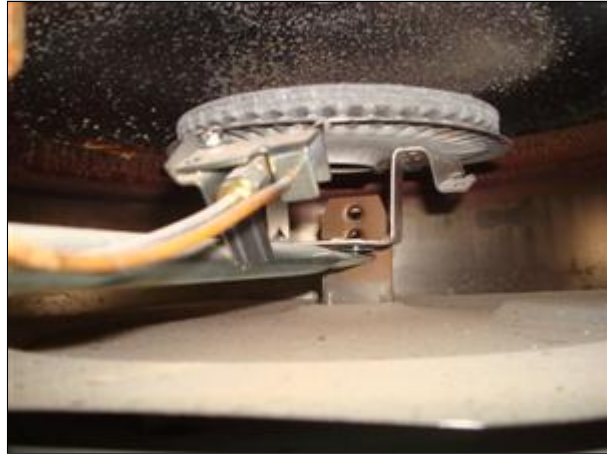
10.4 Picture 2 View of combustion chamber.
