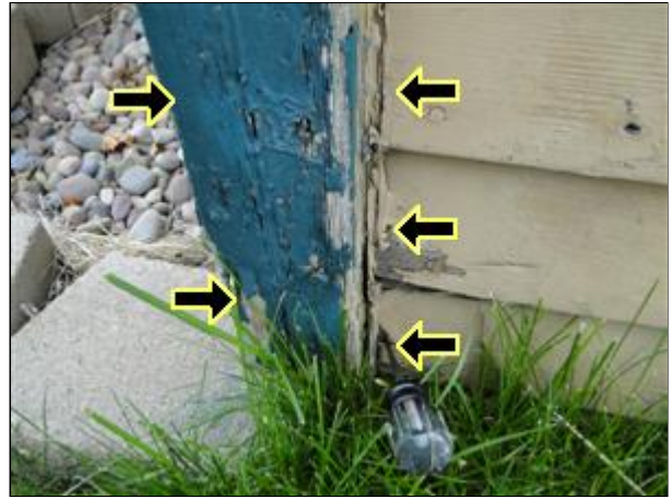
2.1 Picture 6 Trim board needs repair and caulking where cladding boards meet.
