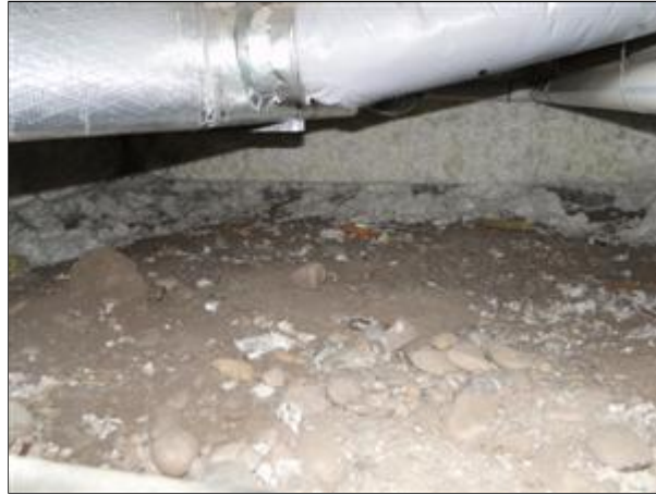
9.4 Picture 1 East crawlspace off of basement does not have vapor barrier.
