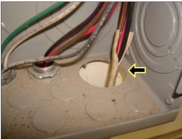
8.8 Picture 2 Knock out missing collar.
