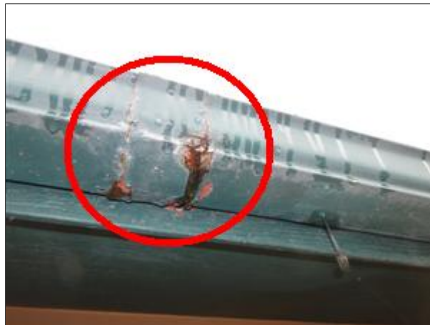
1.4 Picture 2 Rust present at joint here.
