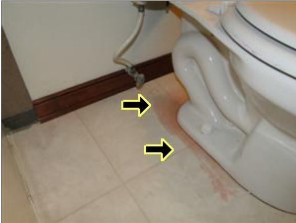
6.13 Picture 1 Standing water here.
