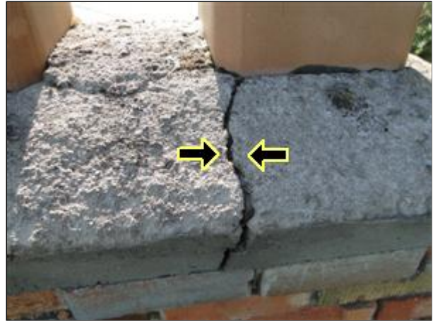
1.2 Picture 5 Crack at chimney cap.
