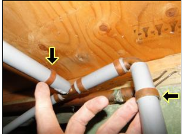
10.1 Picture 2 Loose clamp fittings at unions here.
