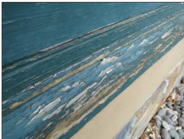
2.2 Picture 2 Close up of damage.
