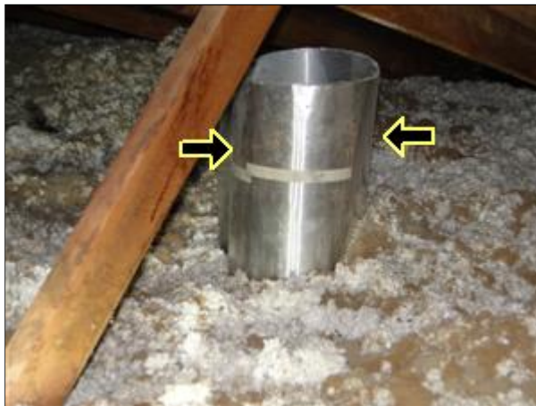
4.6 Picture 1 Duct work terminates in attic.
