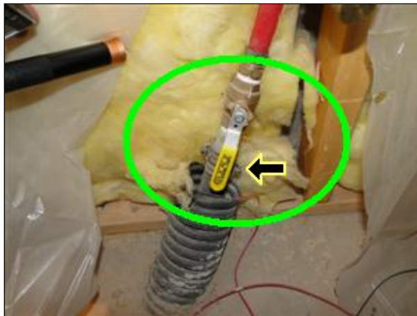
10.3 Picture 1 Water main shut off valve.
