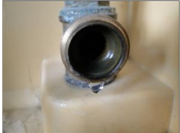
10.11 Picture 2 Close up of drip leak at hot water faucet.
