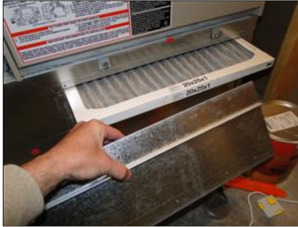
11.4 Picture 1 Filter located behind this panel.
