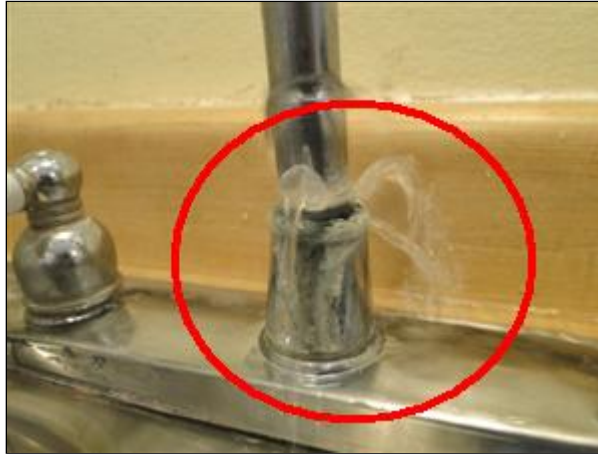
5.10 Picture 1 Leak at swivel neck.
