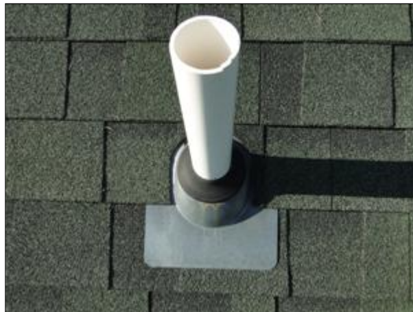
1.2 Picture 1 Vent stack installed correctly.
