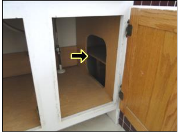
6.16 Picture 2 Spa access panel under cabinet.
