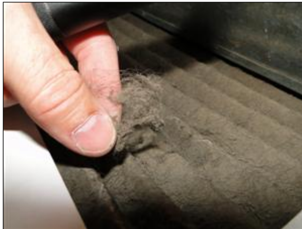
11.4 Picture 2 Filter is really dirty.
