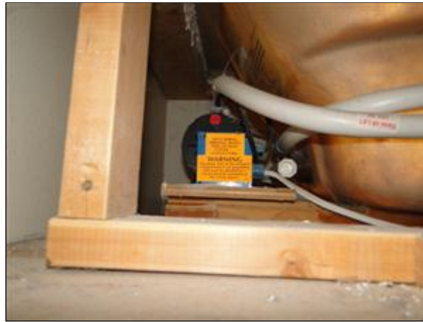
6.16 Picture 3 View inside access area and pump.
