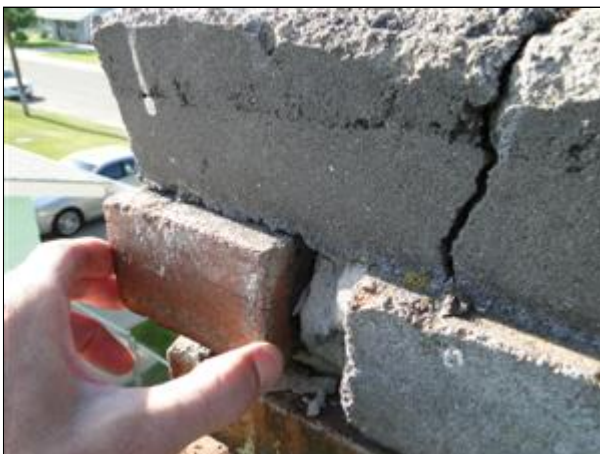
1.2 Picture 8 Loose corner bricks, crack at cap.
