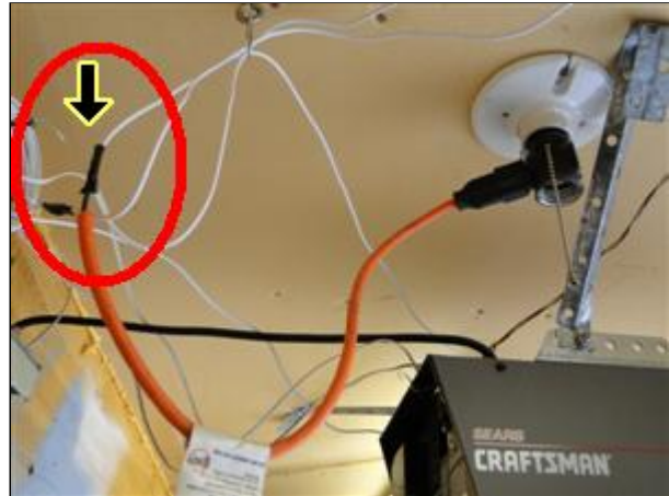
3.7 Picture 2 Orange extension cord with open air splices for light fixtures.
