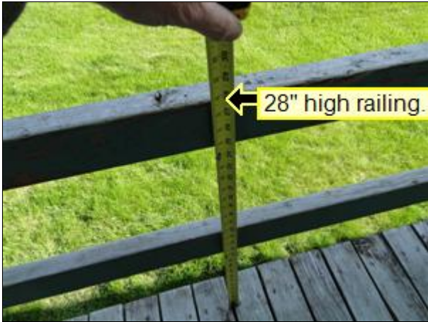
2.4 Picture 5 Railing way too short.
