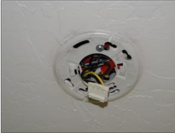
7.8 Picture 1 Missing smoke detector at master.
