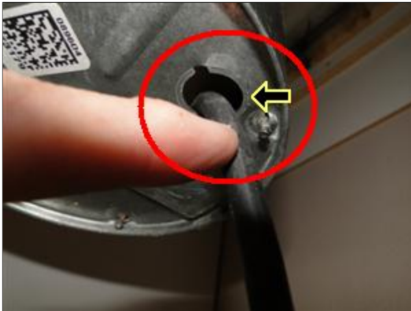
5.12 Picture 1 Collar missing here.
