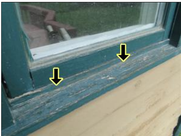
2.2 Picture 1 Maintenance needed htere.
