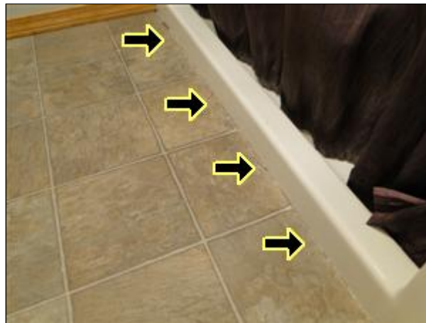
6.16 Picture 4 Caulking missing or failing here.
