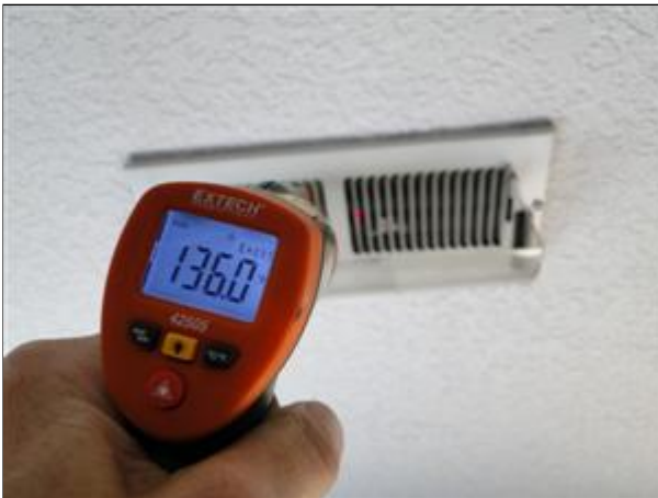
11.0 Picture 3 136 at upstairs ceiling vents.
