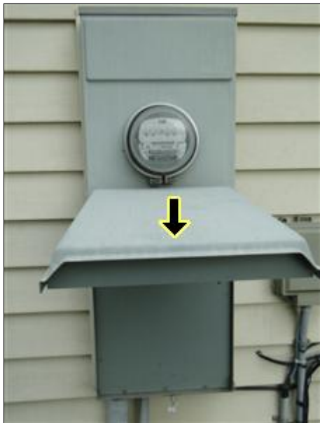
8.1 Picture 1 Main breaker under this panel.
