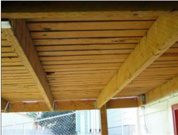
2.4 Picture 3 Floor joists spaced to far apart, run wrong direction.
