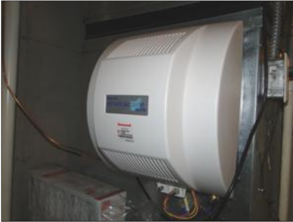
11.0 Picture 5 View of humidifier.
