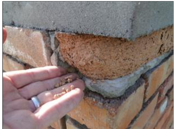
1.2 Picture 7 Corner bricks crumbling.
