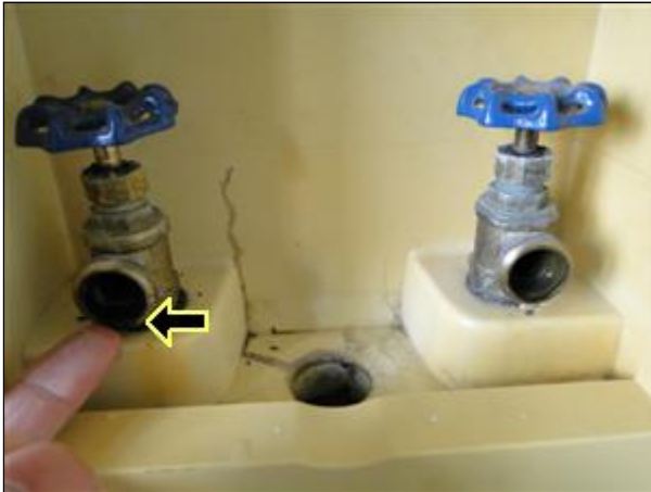
10.11 Picture 1 Drip leak here.
