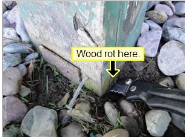
2.4 Picture 4 Rot at support post, earth to wood contact.
