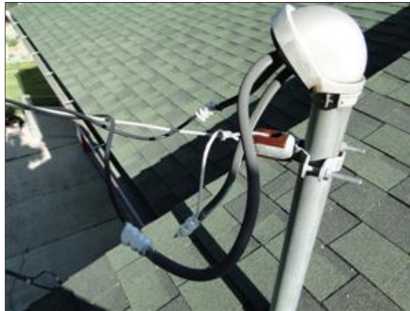
8.0 Picture 1 Overhead mast for entrance conductors.
