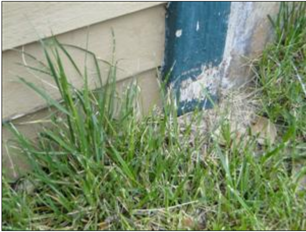
2.1 Picture 5 Earth to cladding and trim contact.
