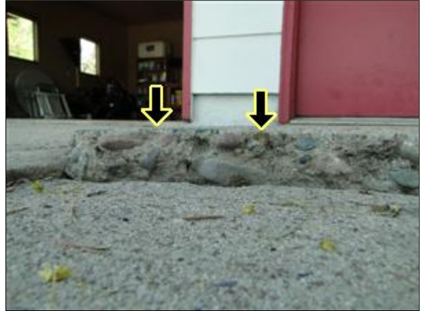
2.11 Picture 2 View of off set concrete, over 2" inches.
