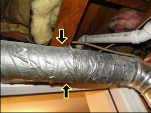
10.12 Picture 2 Completely wrapped in duct tape indicates issues.
