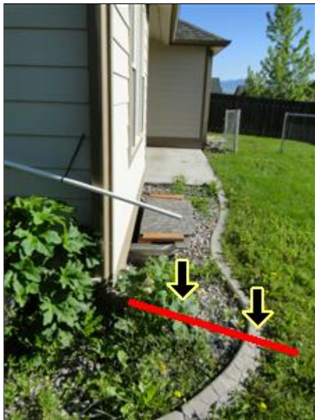
1.5 Picture 2 Downspout extension needed here to lawn area.
