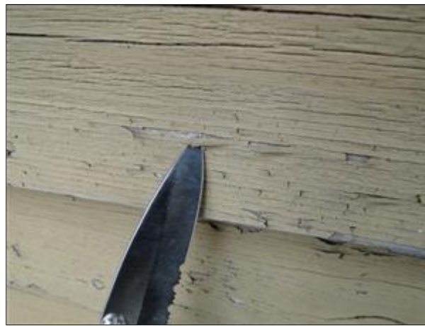
2.1 Picture 7 Peeling paint, checking cladding boards.
