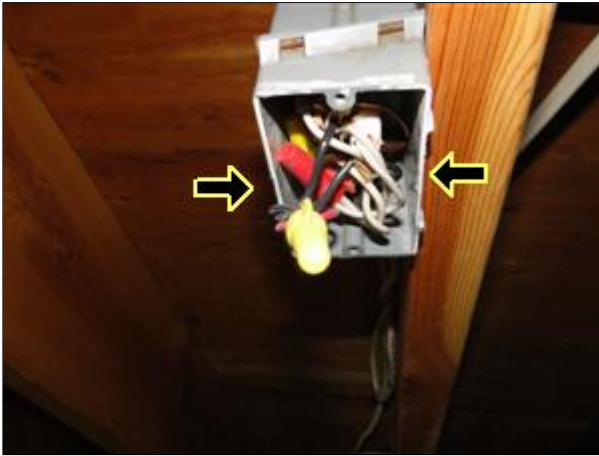
9.13 Picture 2 Open junction boxes at basement.
