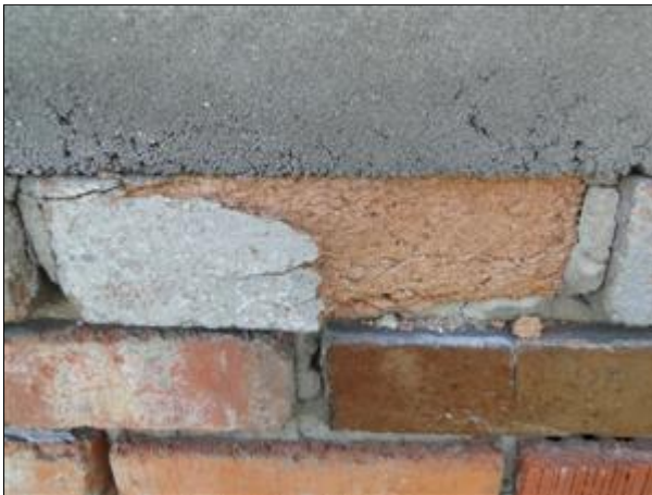
1.2 Picture 6 Bricks starting to decay.
