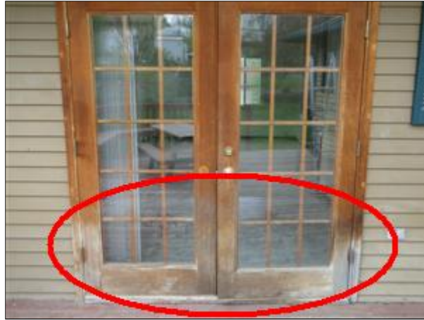
2.3 Picture 1 Wood finish at door failing here.
