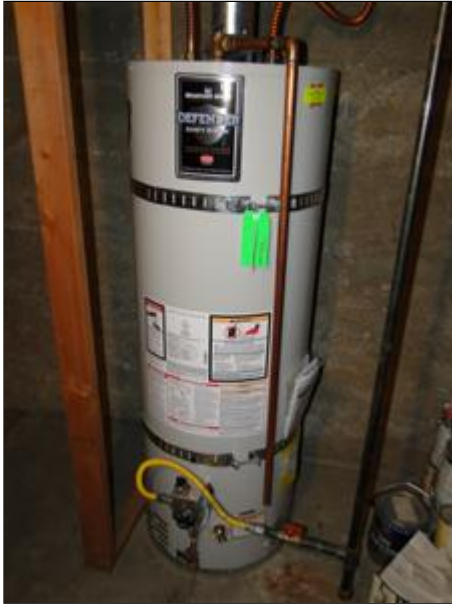
10.4 Picture 1 View of water heater.
