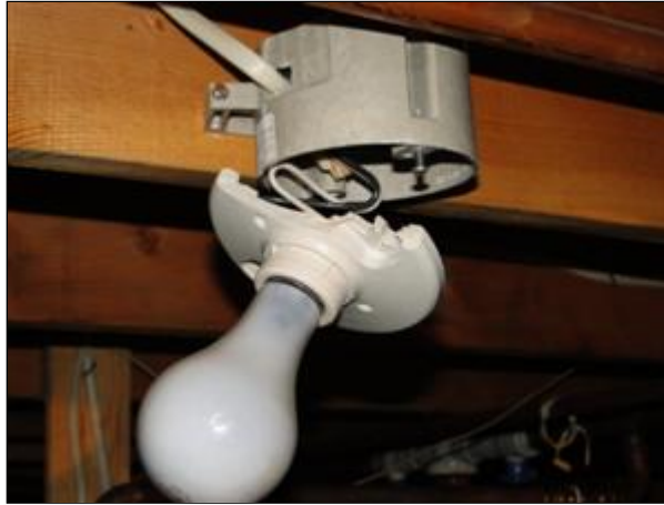
9.13 Picture 1 Porcelain light fixture damaged.
