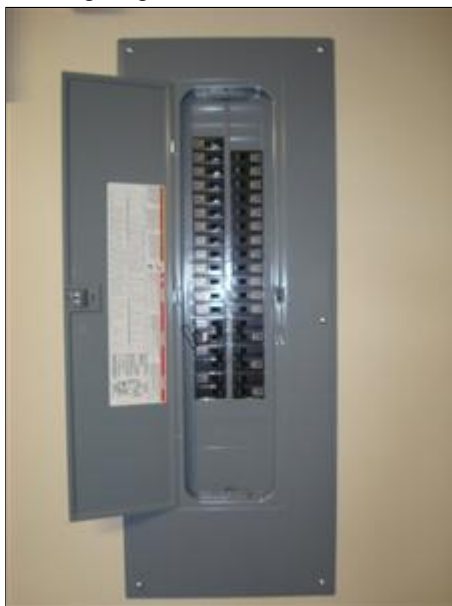
8.2 Picture 1 Main breaker box.
