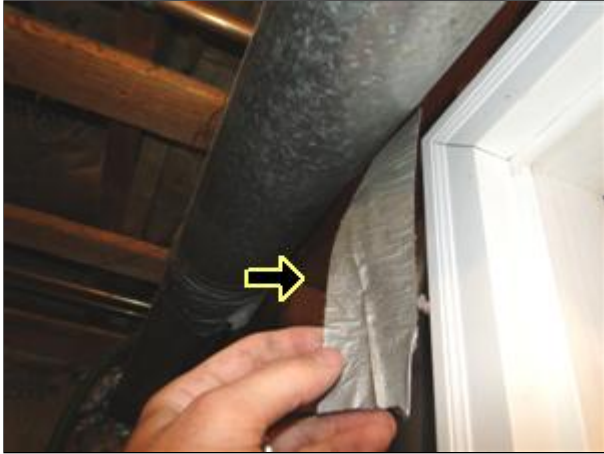
10.12 Picture 3 Duct tape delaminating at joints.
