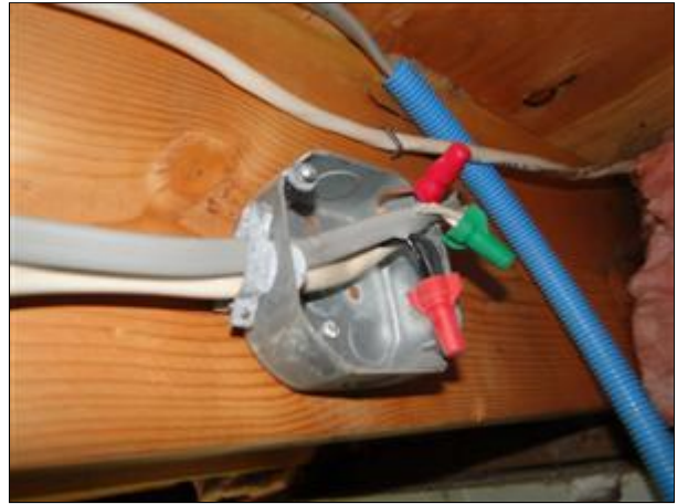
9.13 Picture 3 Open junction box.
