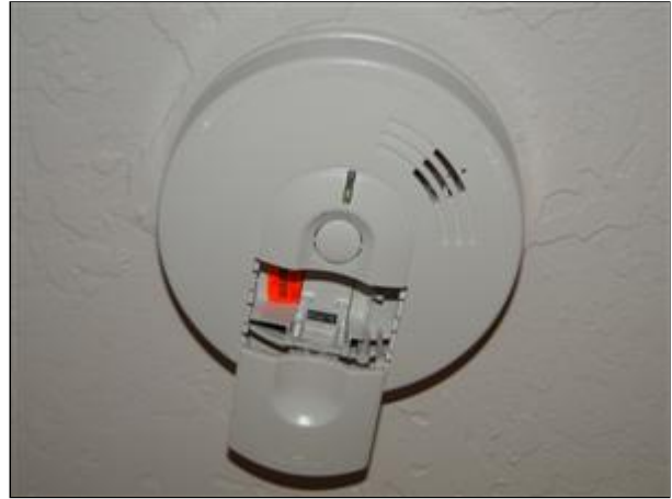
7.8 Picture 2 Most detectors are missing back up batteries.
