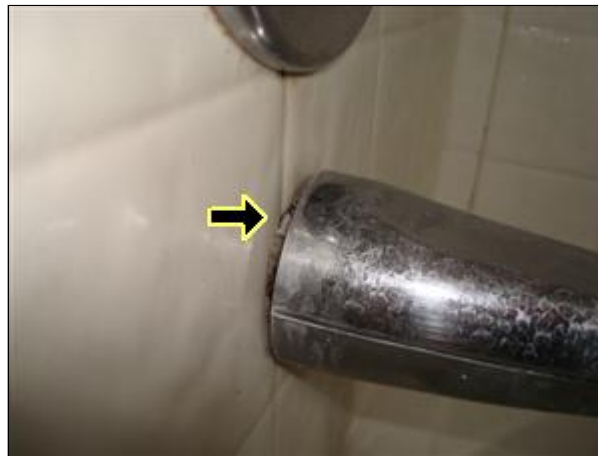
6.15 Picture 1 Gap here needs caulking.
