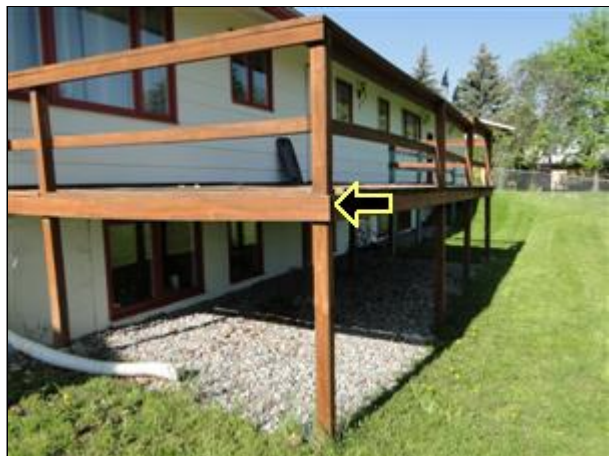
2.4 Picture 10 Push right here, whole deck sways.
