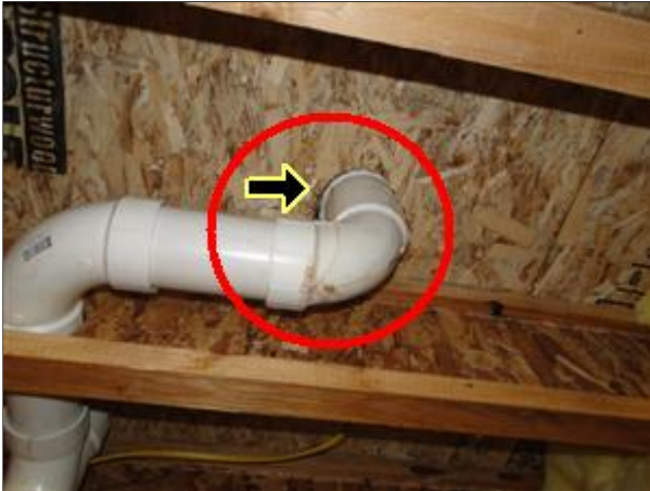
10.0 Picture 1 Leak located here.
