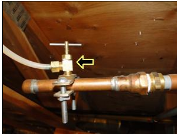
10.1 Picture 3 Saddle valve, not good.
