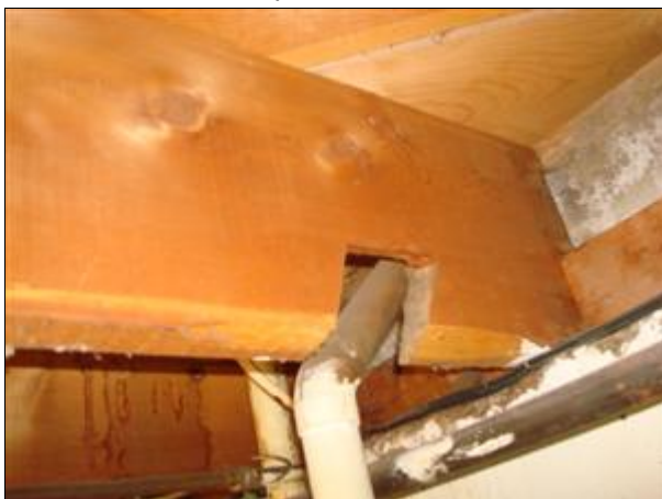
9.2 Picture 1 Joist over notched.
