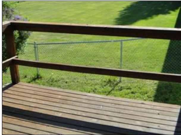
2.4 Picture 6 Spindles missing at railing.
