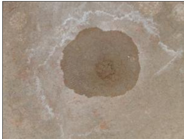
10.0 Picture 3 Wet spot at floor with previous stain marks.
