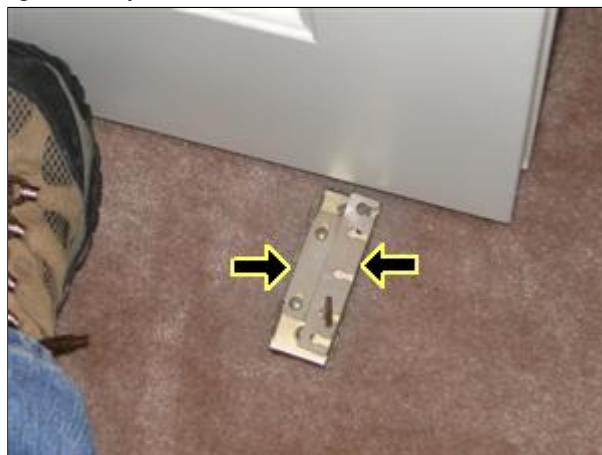
7.7 Picture 1 Door guides missing at bedrooms.
