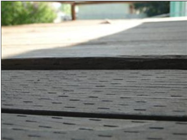
2.4 Picture 7 Trip hazard at deck boards.
