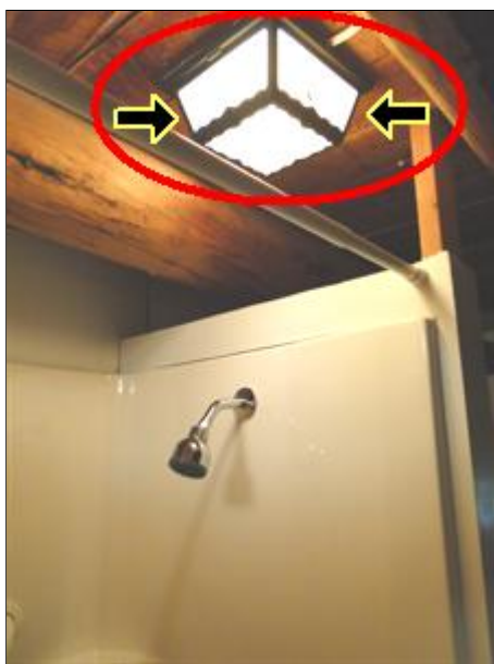
6.7 Picture 1 Shock hazard at light fixture.
