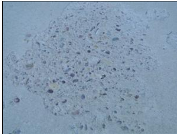
2.11 Picture 3 Spalling, exposing aggregate.
