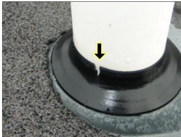
1.2 Picture 10 Cracks in rubber sleeve.
