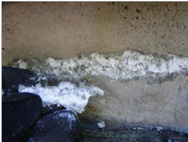
2.5 Picture 2 View of north foundation and white powdery substance.
