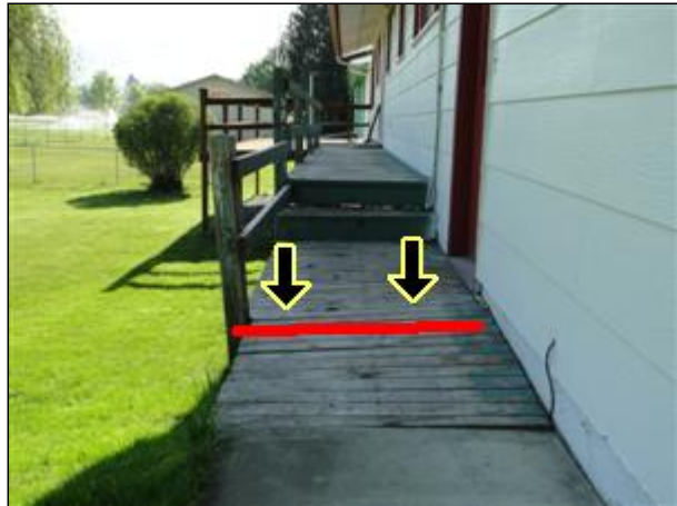
2.4 Picture 8 Deck walk way tilted.
