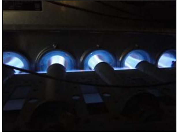
11.0 Picture 2 View of burners.
