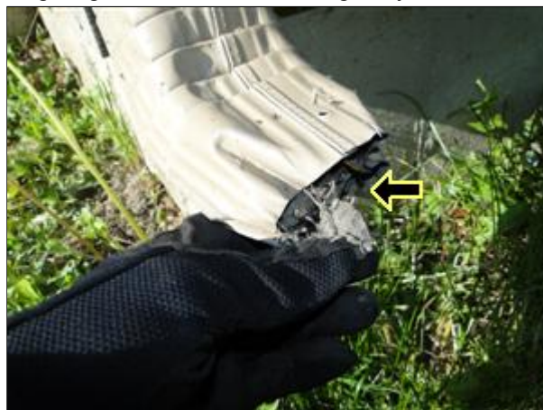
1.5 Picture 1 Downspout clogged here.
