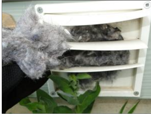
10.12 Picture 4 Dryer vent hood completely blocked.
