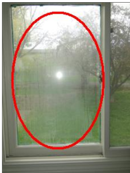
7.5 Picture 1 Broken seal this window.
