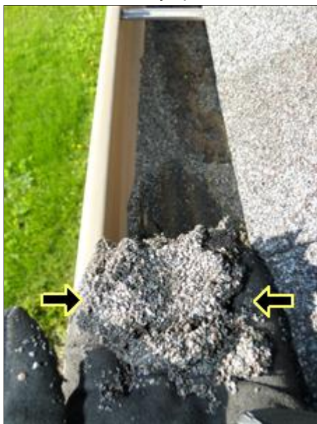
1.4 Picture 1 Handfull of granules from gutter.
