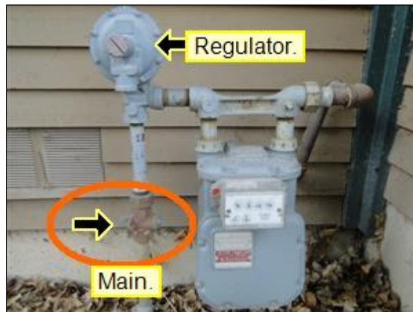
10.10 Picture 1 Main gas shut off valve.
