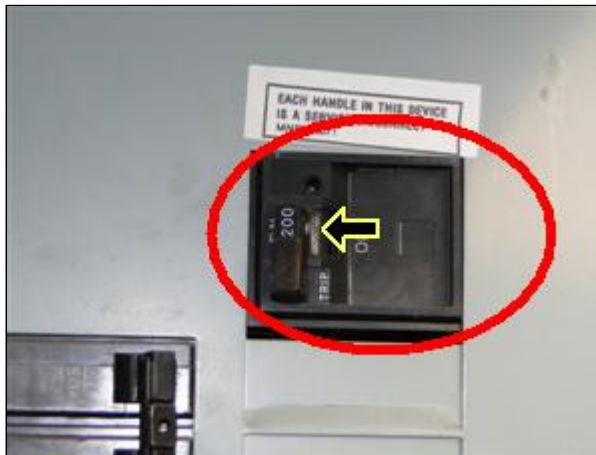
8.1 Picture 2 View of main breaker.
