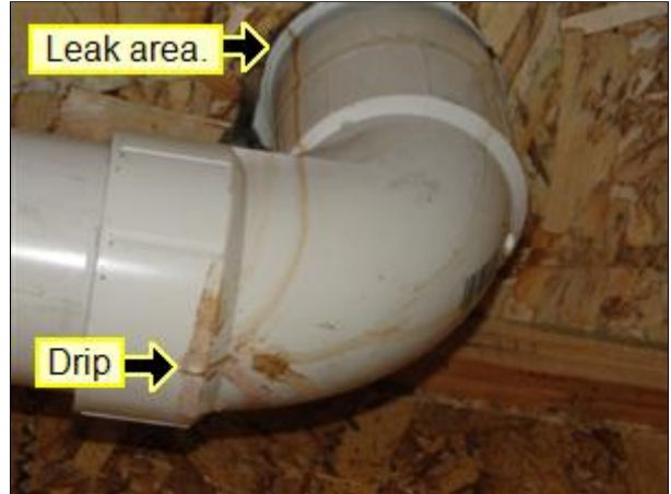
10.0 Picture 2 Close up of leak.
