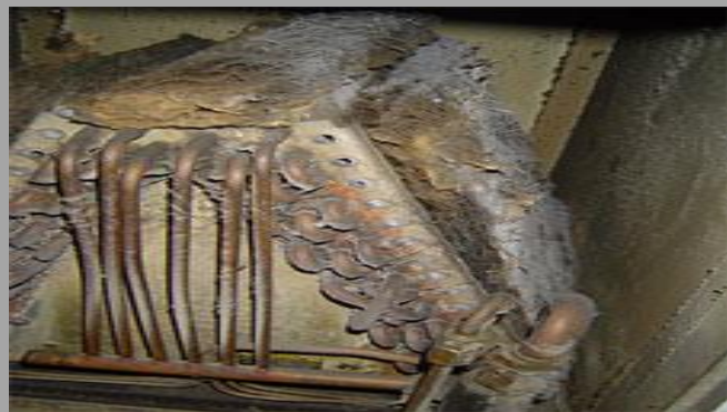
Figure 1: Dirty Air Coil
