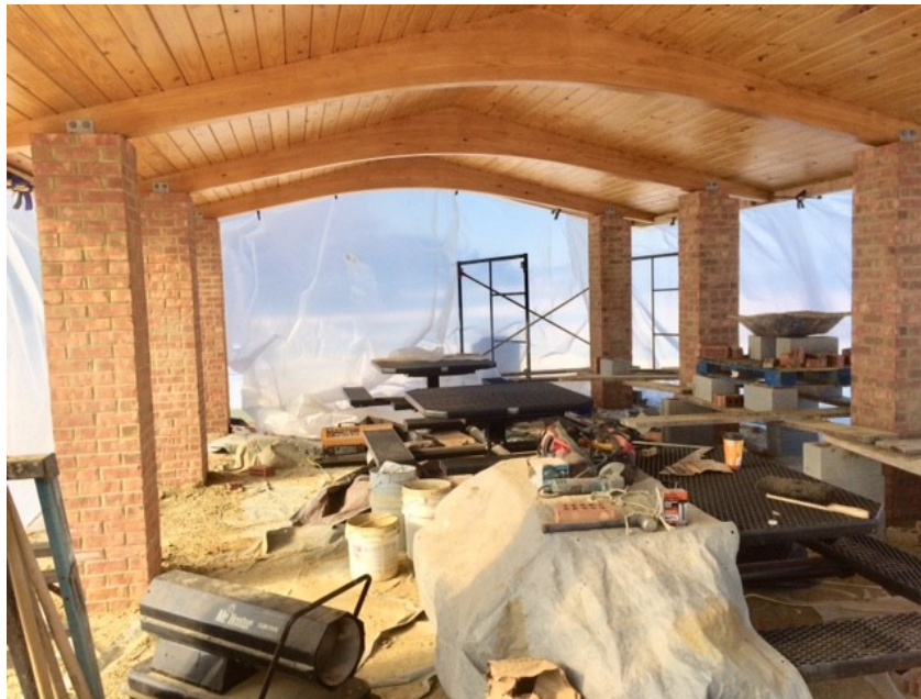
The masons worked through a week of freezing temperatures by enclosing structure in plastic sheeting - they should finish in coming week of January 8-17.
