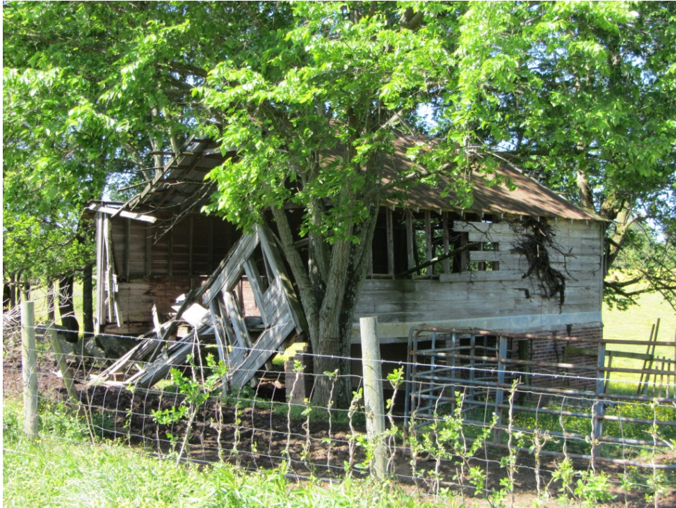
Figure 28. NCDOT Survey #9, Andrew Gibson Farm (GF-0585), 7282 Burlington Road, Guilford County, view of deteriorated secondary residence, looking southwest.
