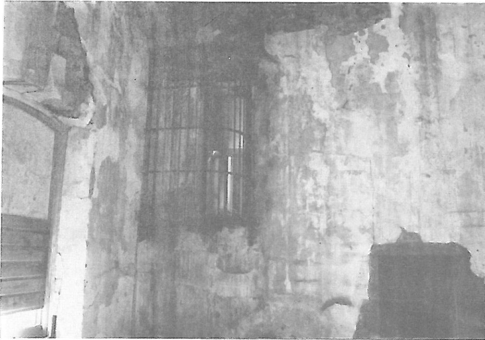
Figure 5: Guard watch station in upper southeast corner of north wing, Wyoming Territorial Prison.
