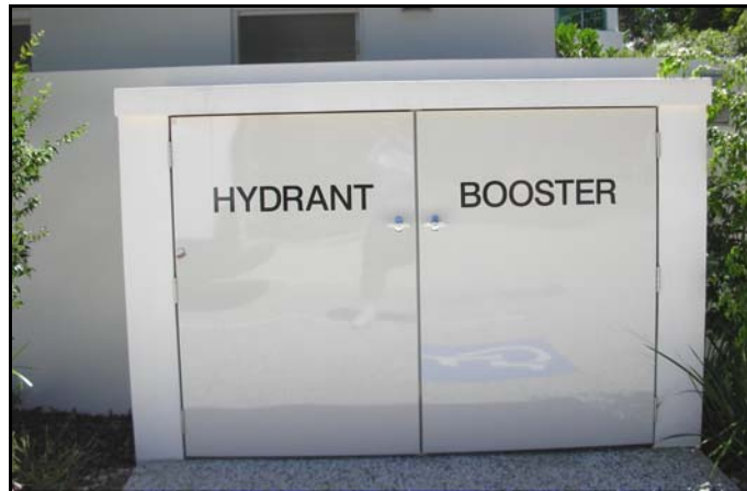
Figure 6– Stainless Steel Booster Cabinet
