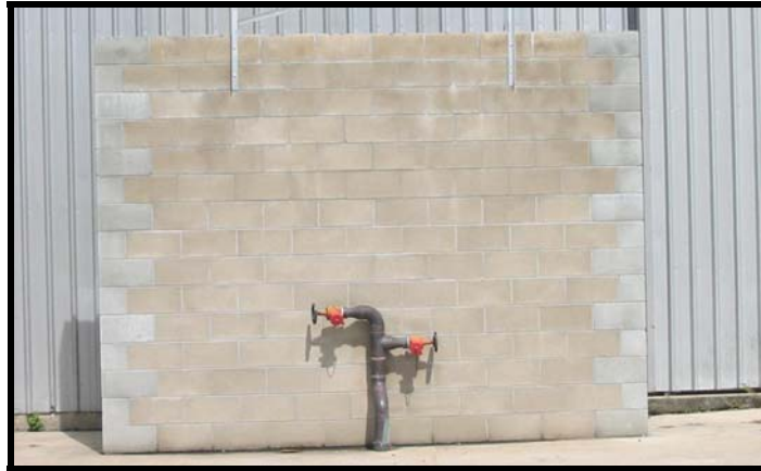
Figure 4 – Protection of External Hydrant
