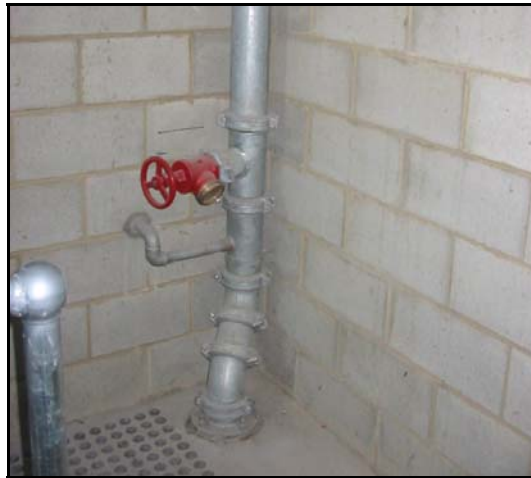
Figure 2 – Hydrant in Fire Isolated Stair
