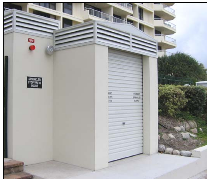
Figure 7 –Enclosure with Roller Shutter – referred to in Coolum Beach as “The Taj Mahal”
