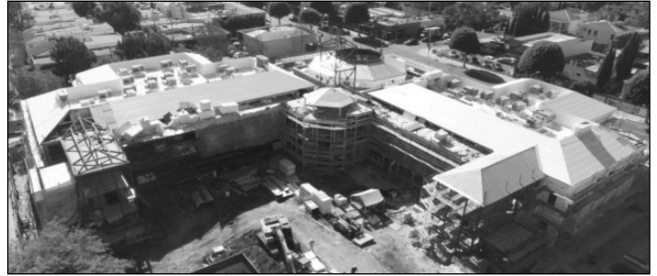
Horace Mann's brand new Building B is nearing completion and is expected to open this fall
