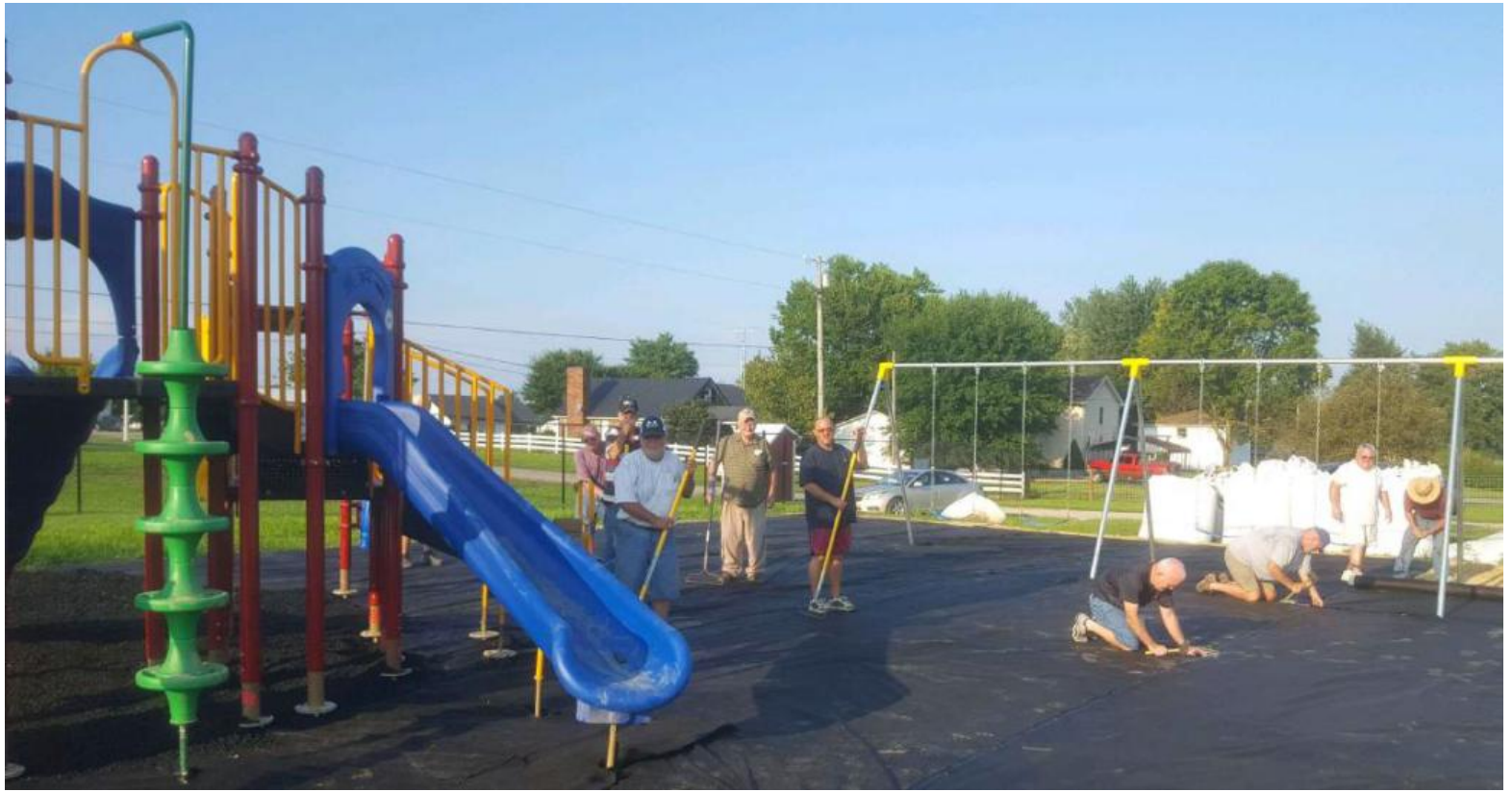
Tollesboro Lions Club members "Work Night" installing filter fabric and mulch on new playground.
