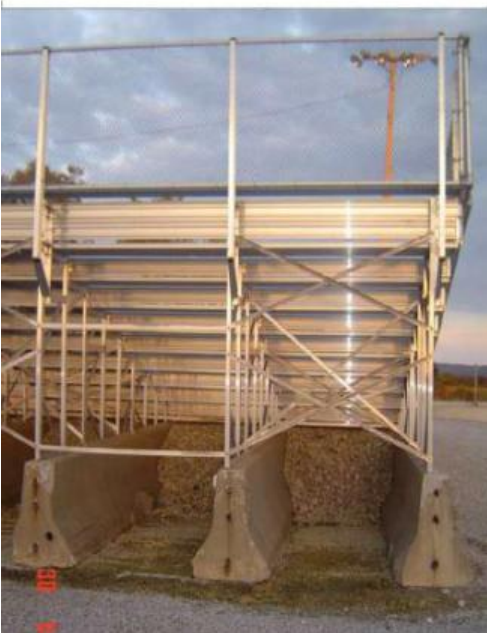
Rear Detail of Elevated Bleacher Set # 1 from the 2009 Grant Application for Bleacher Set # 2.
