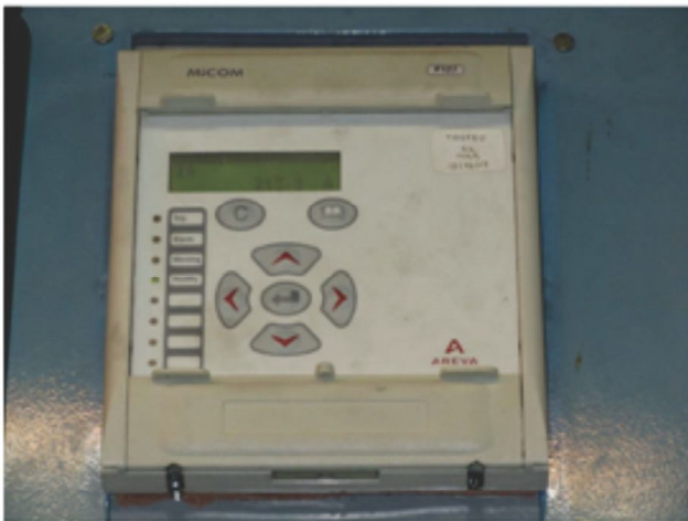
Fig. 5 (Photos—Protection Relays—old & New)
