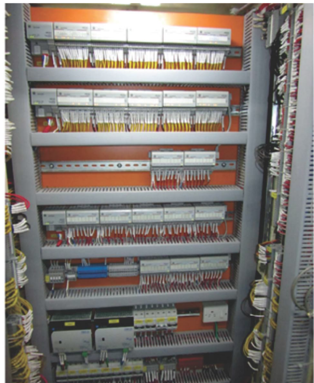
Fig. 6 (Photos—LMS I/O racks—old & New)
