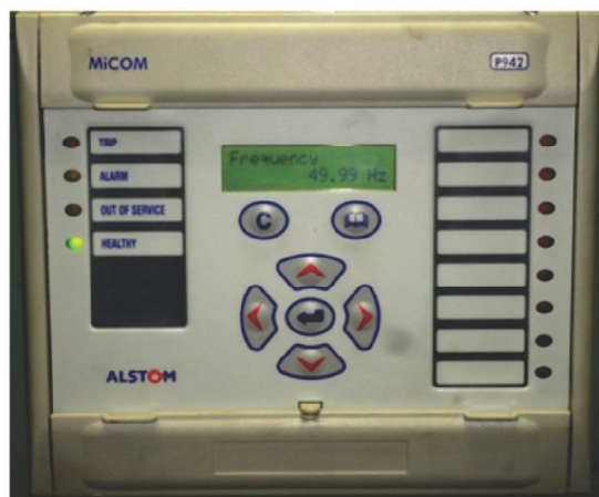
Fig.3 (Photo—Under Frequency Relay)
