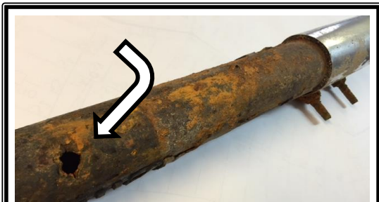
Replaced section of the old 2" steel pipe with hole and previous repair clamp.
