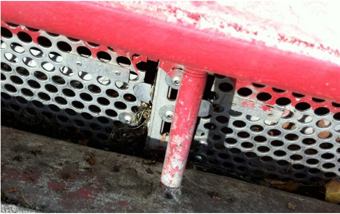
The above two photographs are of the same City of Los Angeles capture device. It has a mechanical clearing mechanism. (Photos taken by Stephen Joseph in Century City on 2-27-12)
