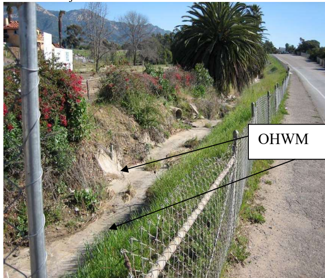
Photo 51. A roadside ditch excavated wholly in uplands, CA. Feature is not jurisdictional under CWA.
