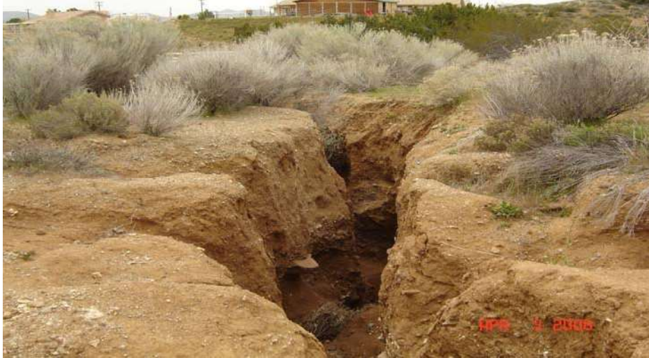
Photo 59: Gullies are eroded channels where surface runoff concentrates. This photo shows a gully formed by eroding material.
