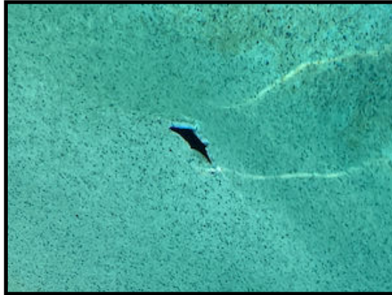
Closer View of Rupture in Finish
