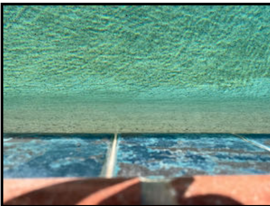
View of Bulge #5
