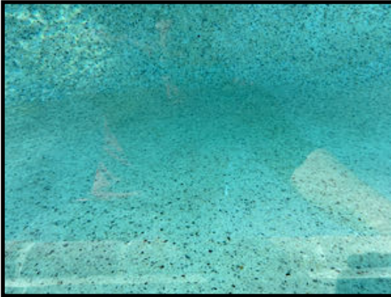
Apparent Calcium Deposit on Bulge in Pool
