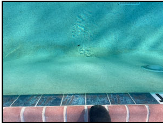
View of Bulge #8
