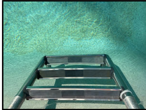
Another View of Pool Wall at Ladder
