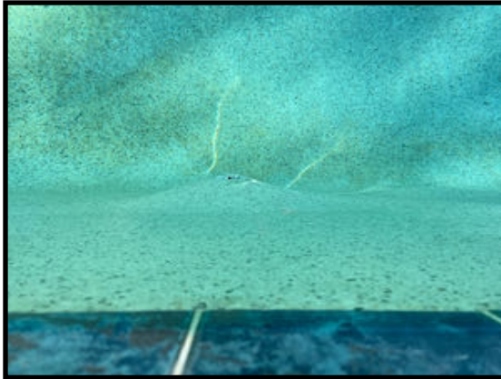
Bulge #7 With Rupture in Finish
