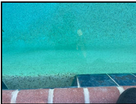
View of Bulge #11
