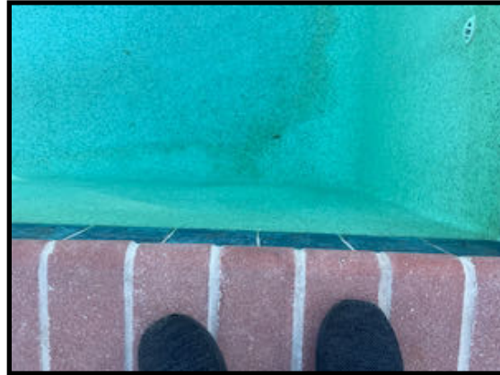
View of Bulge #10
