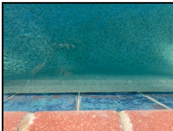
View of Bulge #2
