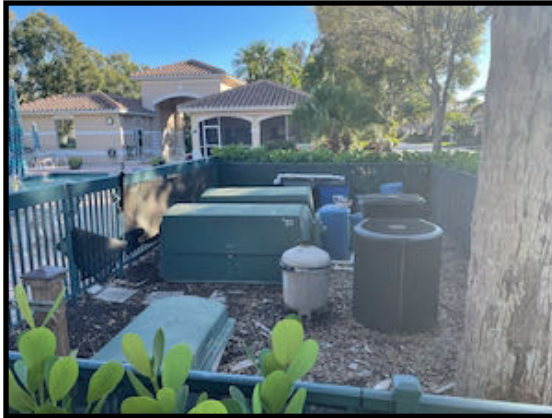
Pool Equipment on West Side of Pool Area
