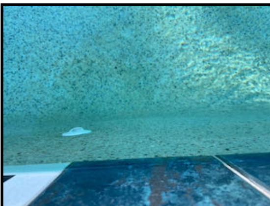
View of Bulge #1
