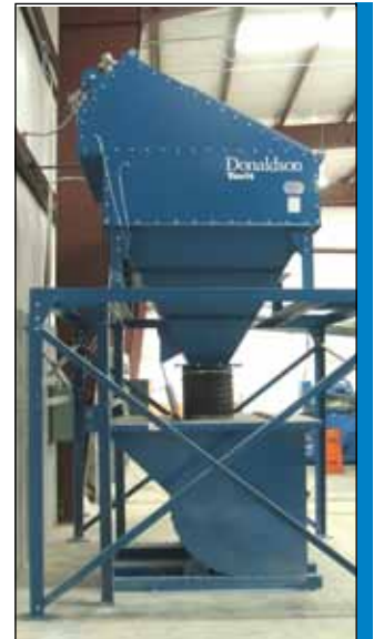
CPV-12 Conveyor line at concrete and asphalt plant (4000 cfm)
