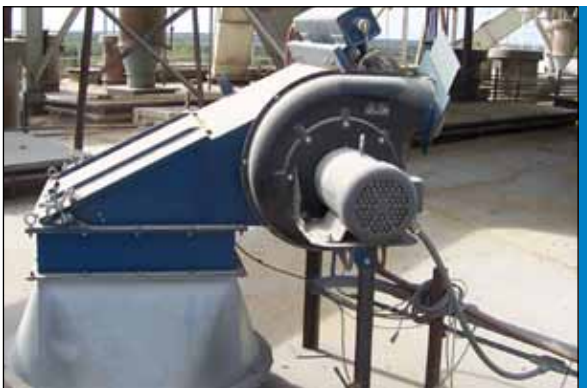
CPV-3 Grain silo bin vent (1200 cfm)
