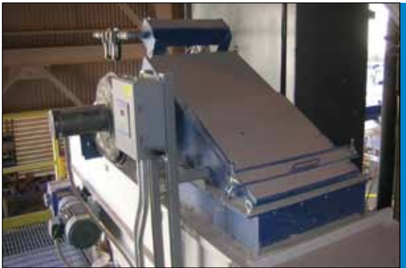
CPV-2 Weigh belt feeder with limestone dust (800 cfm)
