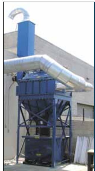
CPV-12 On wood dust at furniture manufacturer (7000 cfm)
