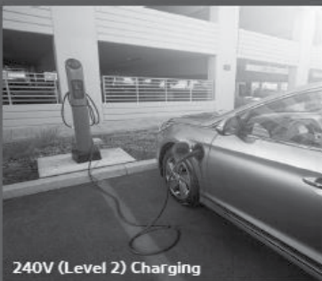
240V (Level 2) Charging
