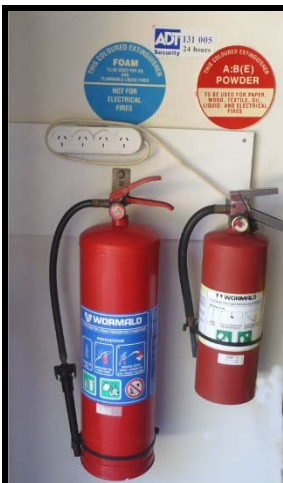
Figure 24 Workshop Fire Extinguishers
