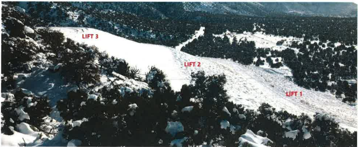
SCA#2 Ash Landfill – west face looking southerly Lift #1 and #2 covered and seeded. Lift #3 in process
